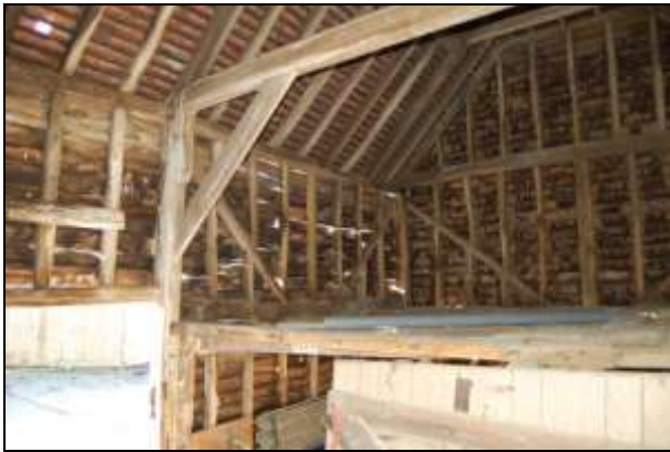
Plate 8: Bay 1: south wall above mezzanine floor
