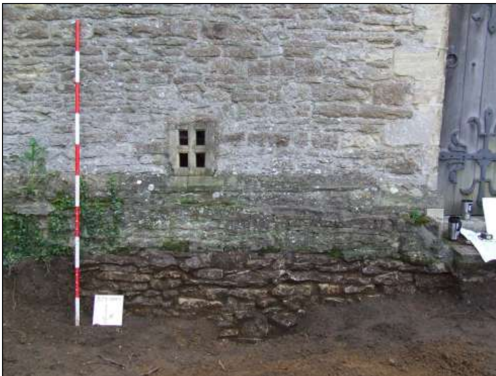
Plate 6: North wall of Church depicting below ground level exposure
