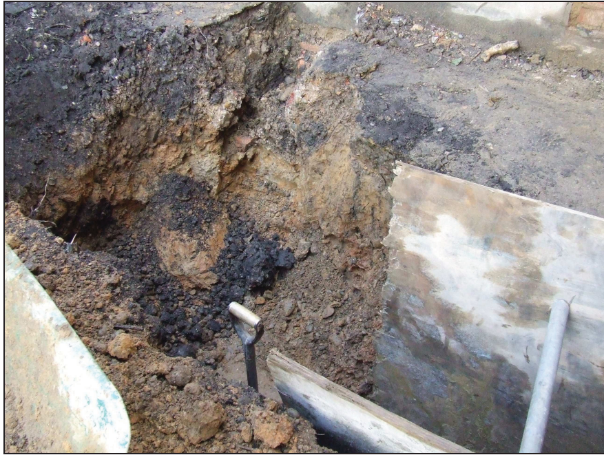
Plate 3: Collapsed trench, looking northwest
