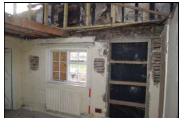
Plate 18: G2, south elevation after removal of ceiling and some walling material, 1m scale
