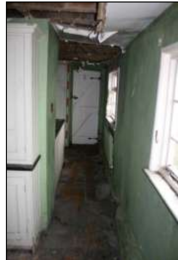
Plate 28: Passageway between G3 and G4, showing reduced sole plate, looking east, 2m scale
