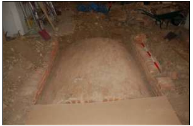
Plate 14: Smith burial vault and brick walls to support the timber floors on either side
