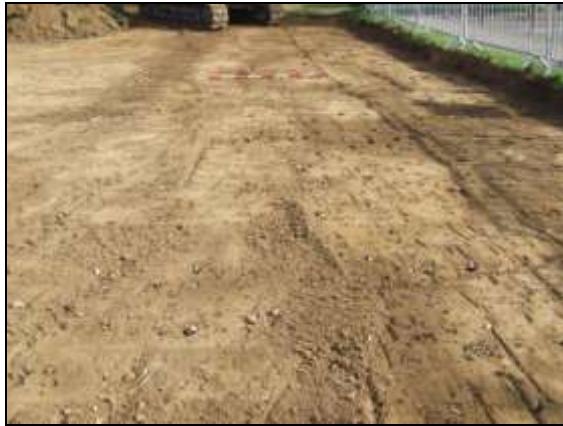
Plate 1: Eastern edge of site, during topsoil strip, looking north east, 2m scale
