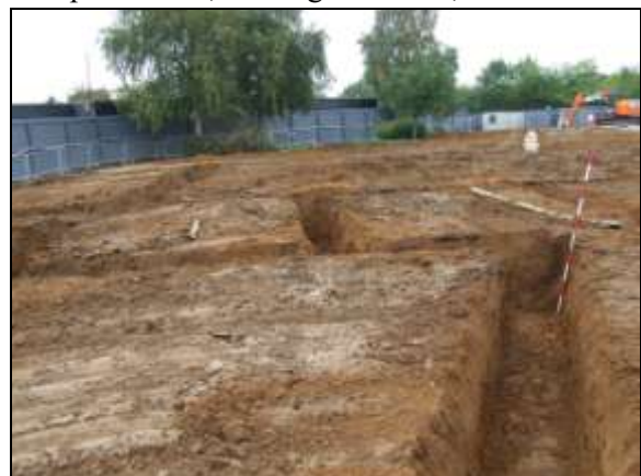
Plate 12: Footing trenches in central part of the site, looking west-south-west, 2m scale
