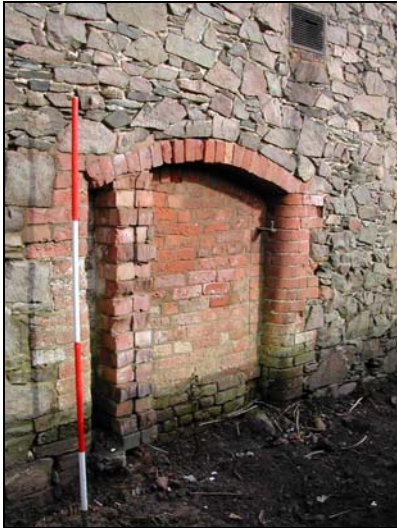
Plate 13: Building 1, blocked door on south side
