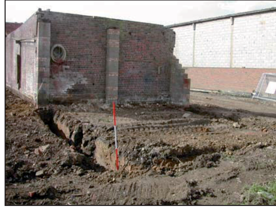
Plate 8: Foundations to the new extension on north side of the old brick building
