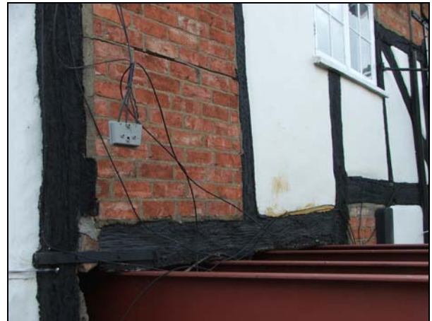
Plate 10: Timber F and wall above repair area
