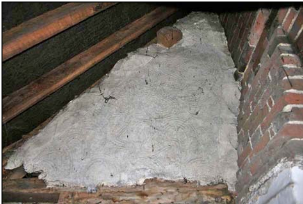
Plate 33: Room F6: plasterwork next to the chimney breast
