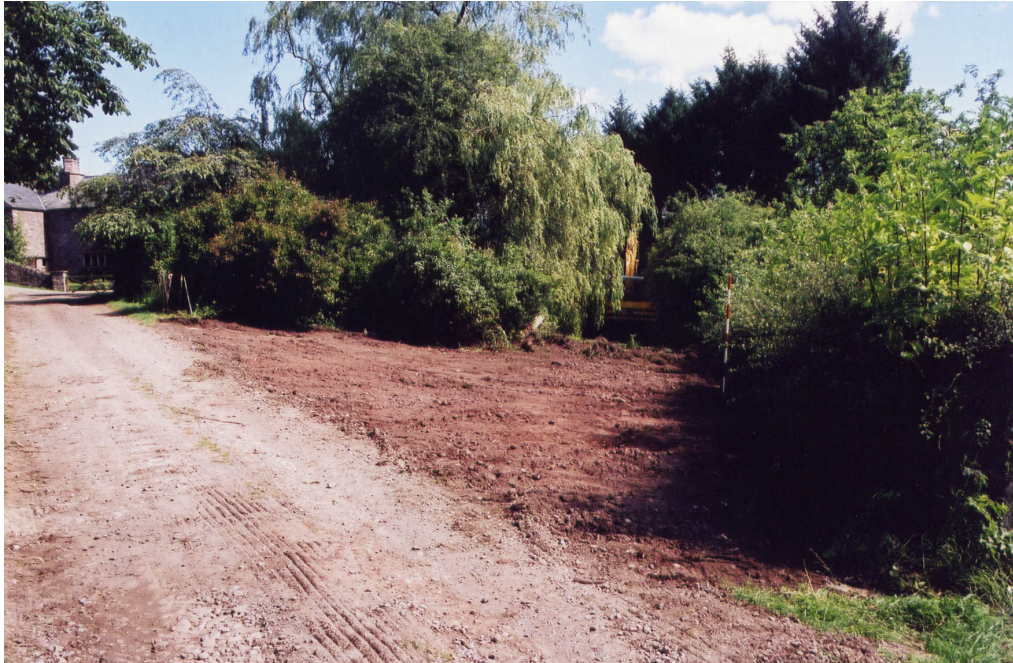
Plate 4: Cleared area for new track way to provide access to swimming pool area
