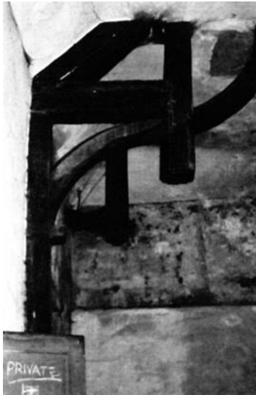
Plate 3: Detail of the hammer beam construction of the roof (provided by The Bromyard History Group)
