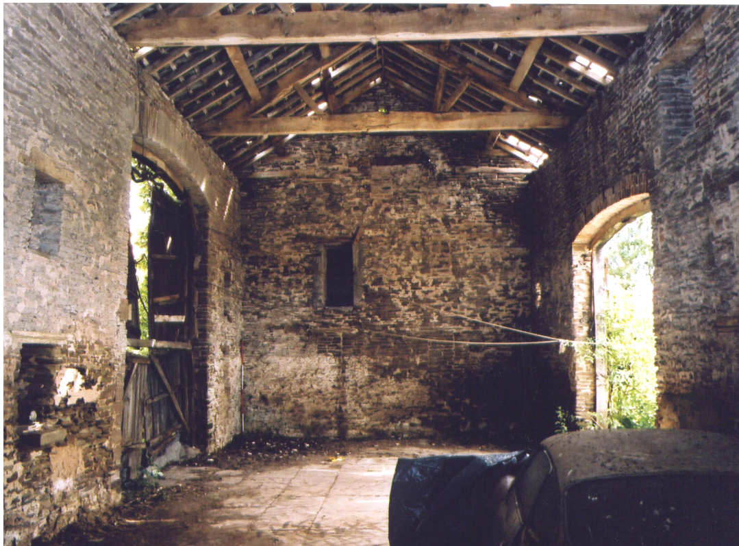
Figure 16: Photograph showing the threshing floor and through-entry. The entrance on the left is higher than the exit on the right.
