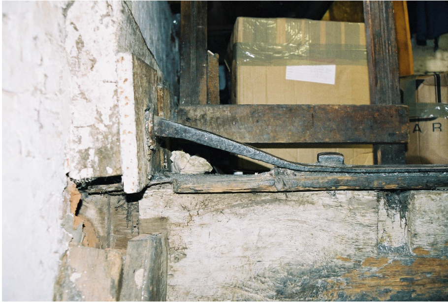
Plate 6: One of three anchorages for the crane built into Building B. Note the spacing plate to the left.
