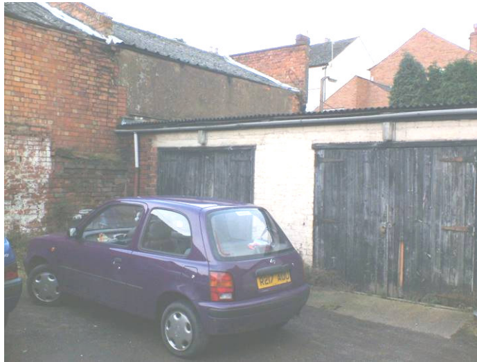
Plate 12: The west elevation of building E and scars of the east-west brick wall
