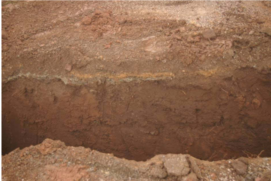
figure 31: tarmac surface and compacted clay base in west-facing section of footpath trench
