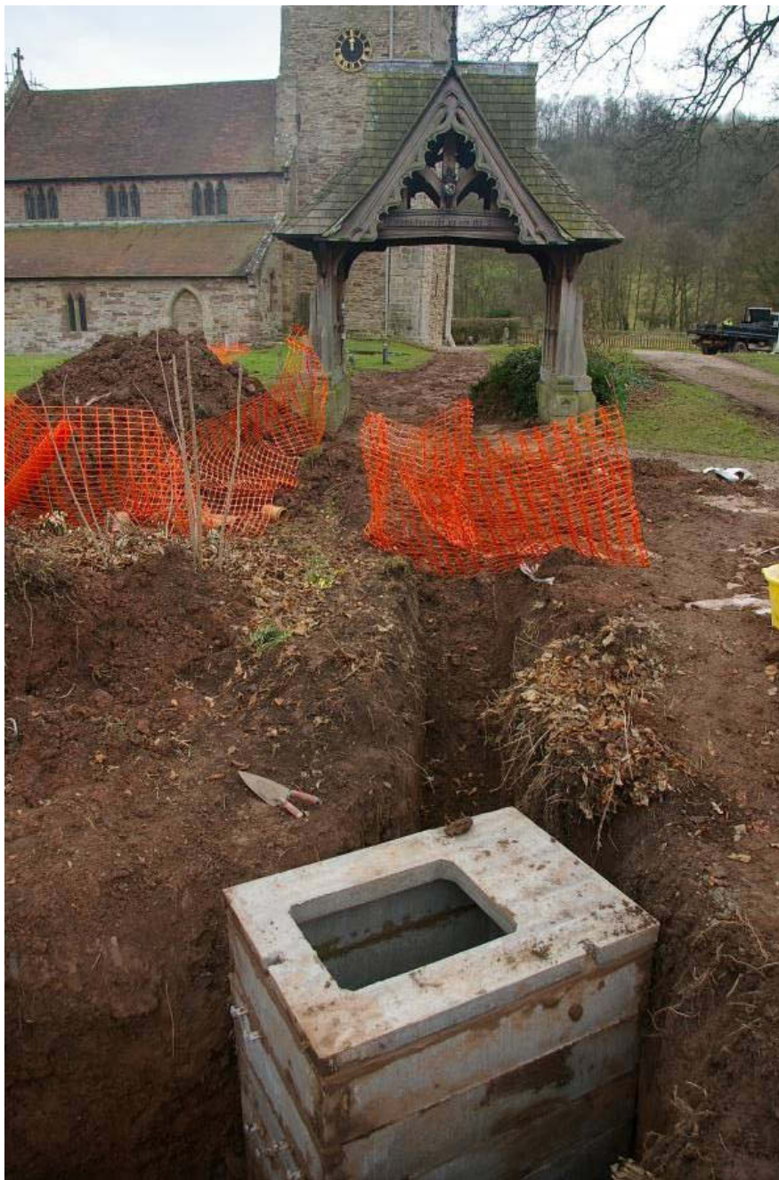
figure 30: looking south from concrete manhole towards the lych-gate and church with previous trenches re-instated.
