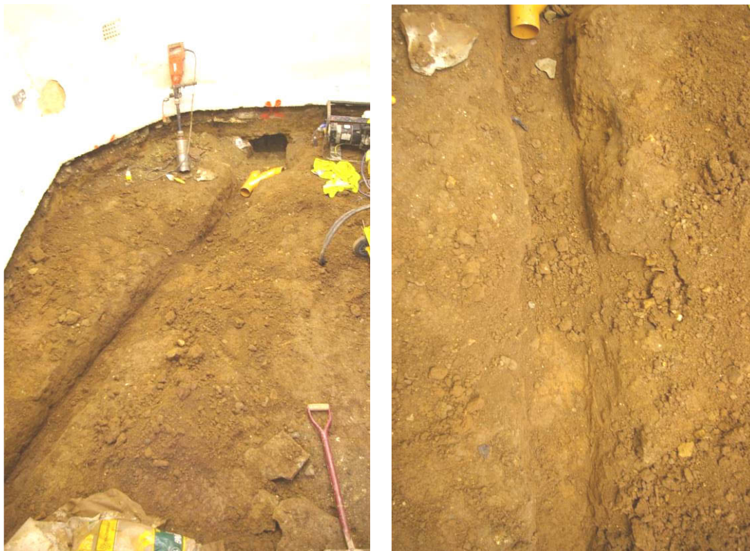
figures 15 and 16: trench for water pipe connection within the church tower, overall and close up
