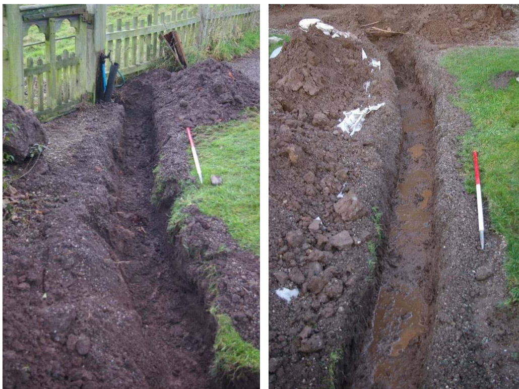
figures 20 and 21: trench connecting water supply to the church, across footpath, looking south-west
