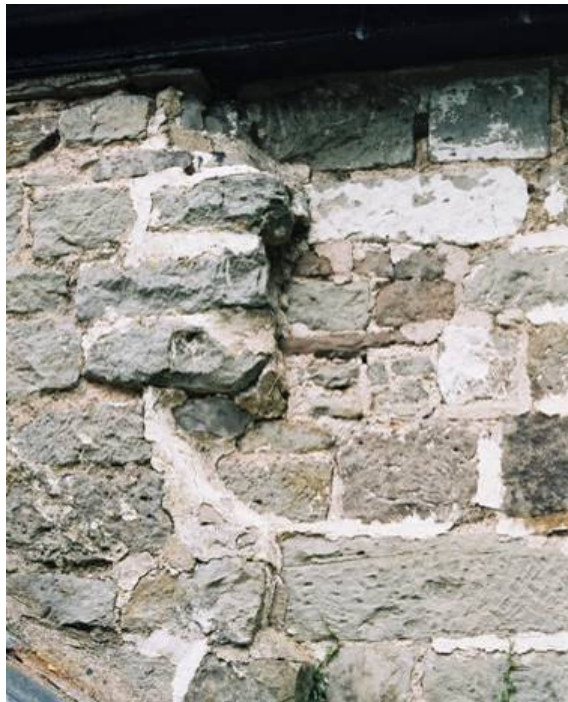
Plate 2: Construction break between the 12 th century wall (east of the door) and the later wall of the Nave
