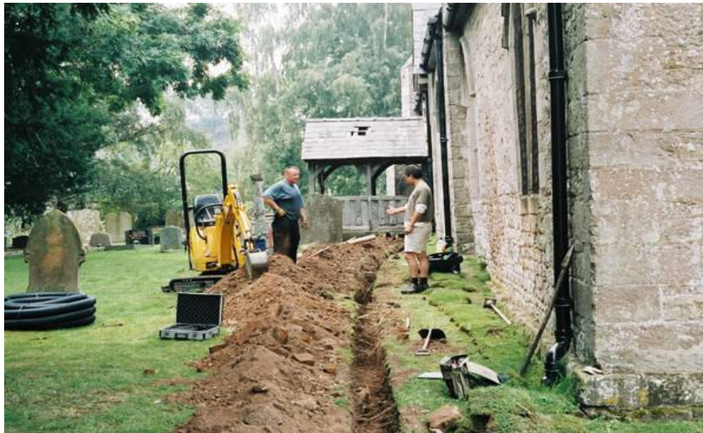
Plate 4: The south trench with the machine by the cut for the manhole
