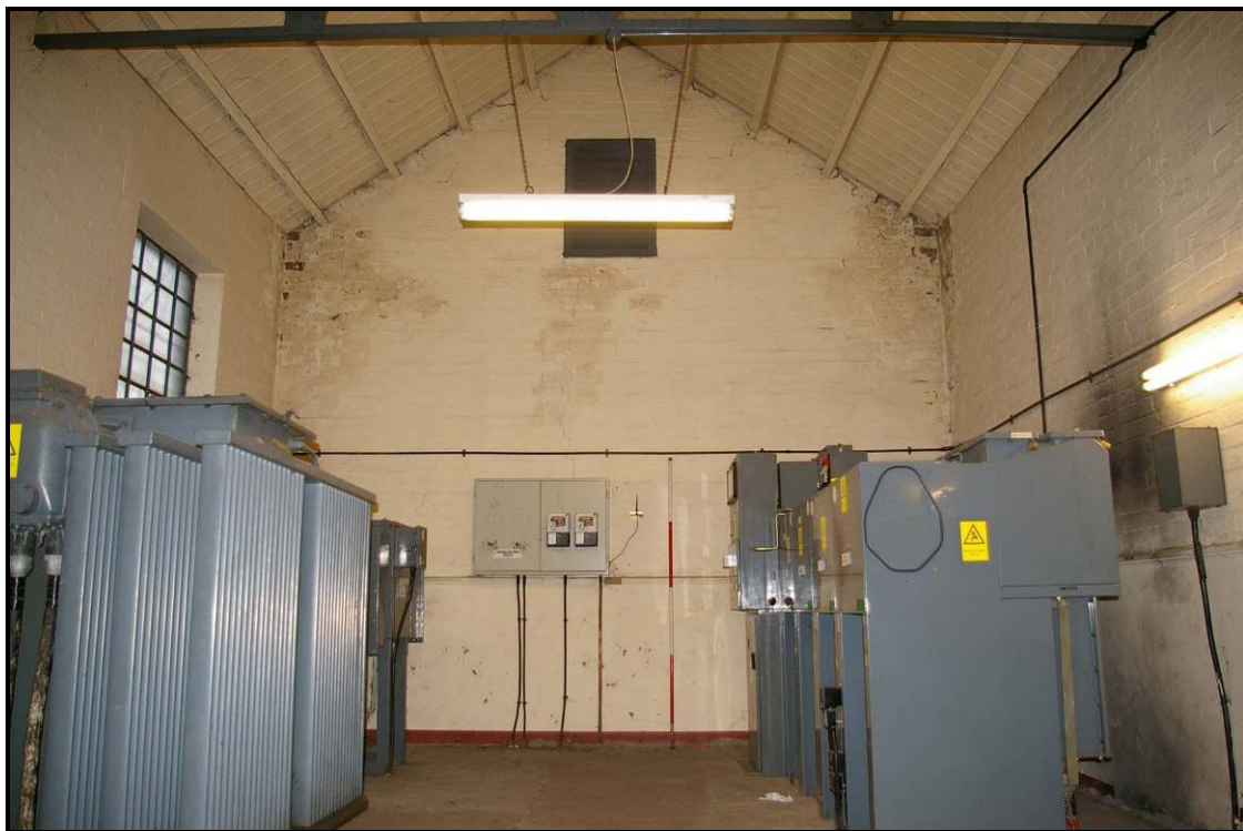
Figure 86: Electrical apparatus inside Building B, looking south
