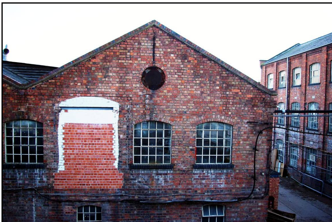
Figure 90: Detail of windows and doorway of former bridge blocked with later bricks
