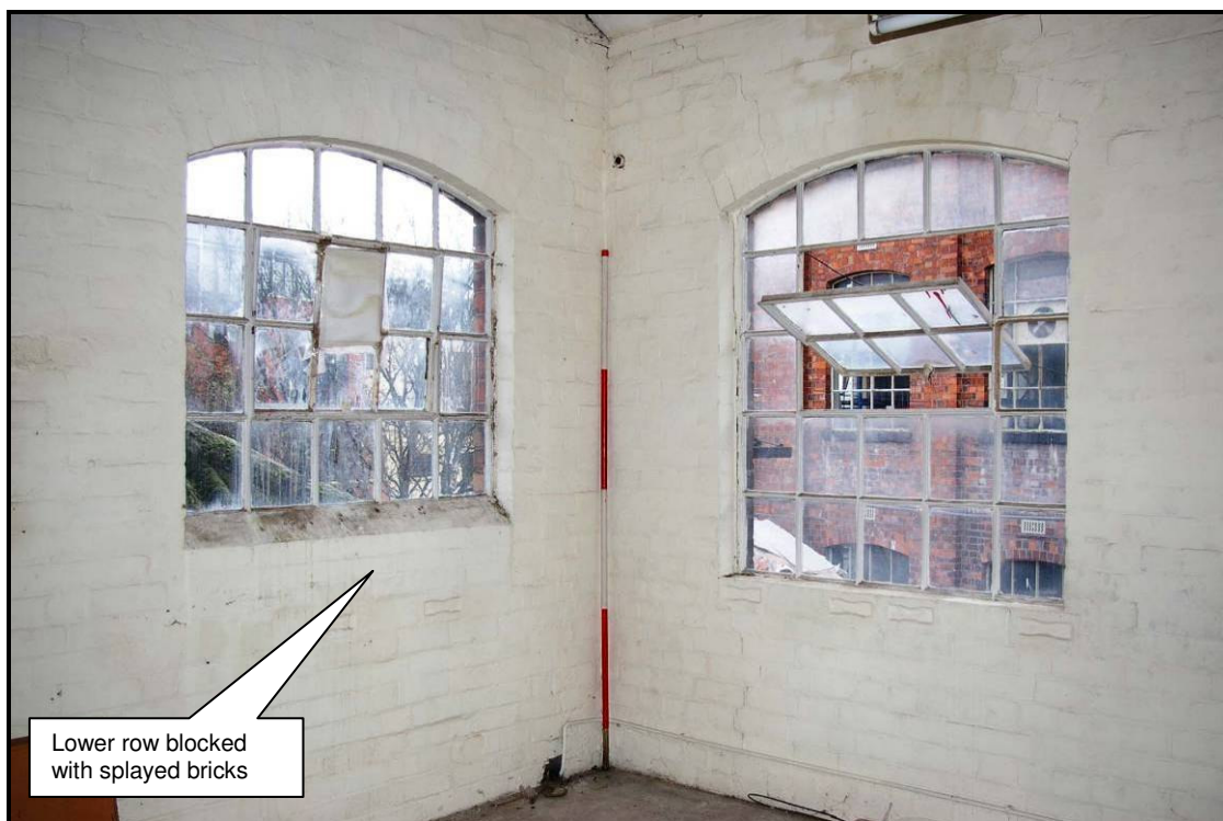
Figure 110: South-east corner of the first floor with modified window on the left
