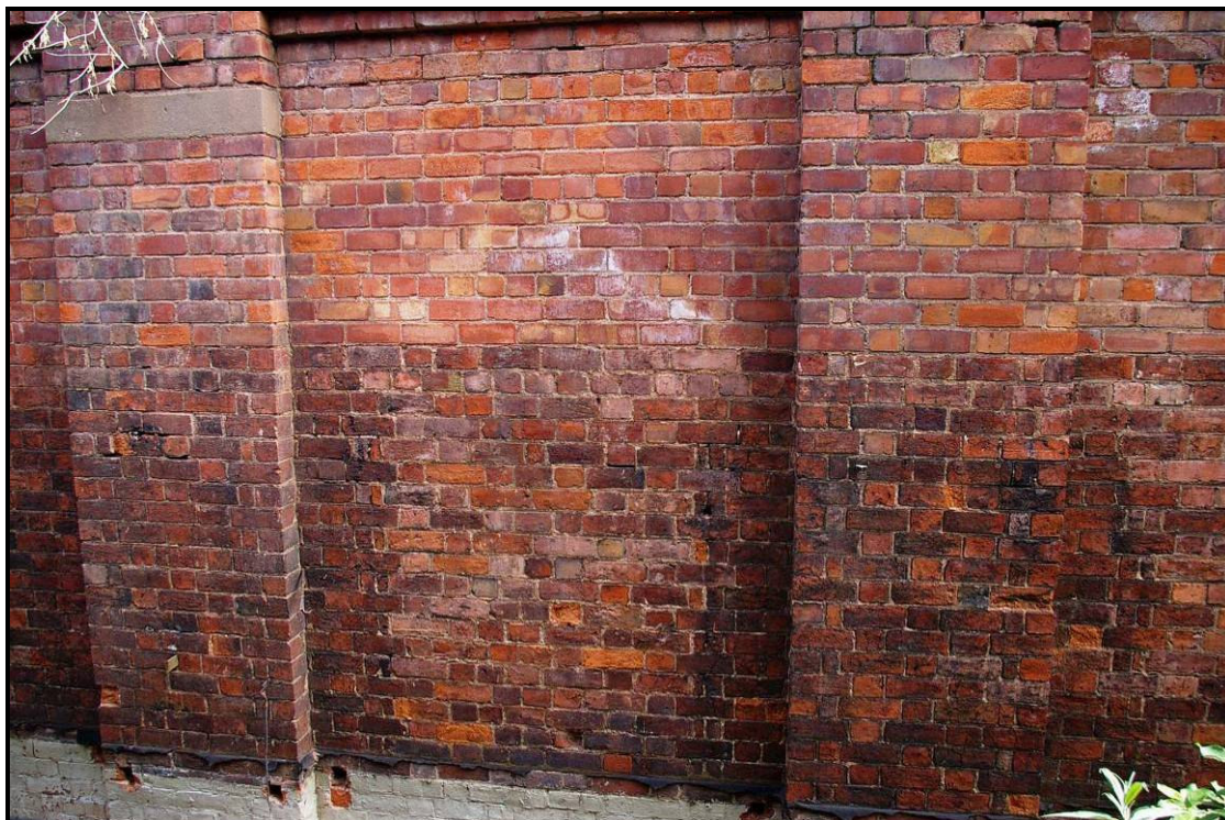
Figure 15: Blocked window on the south elevation
