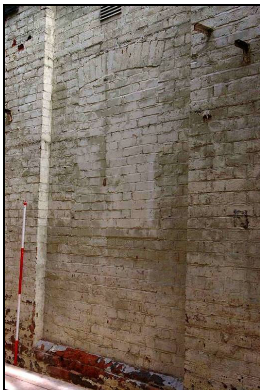
Figure 10: Example of a blocked window
