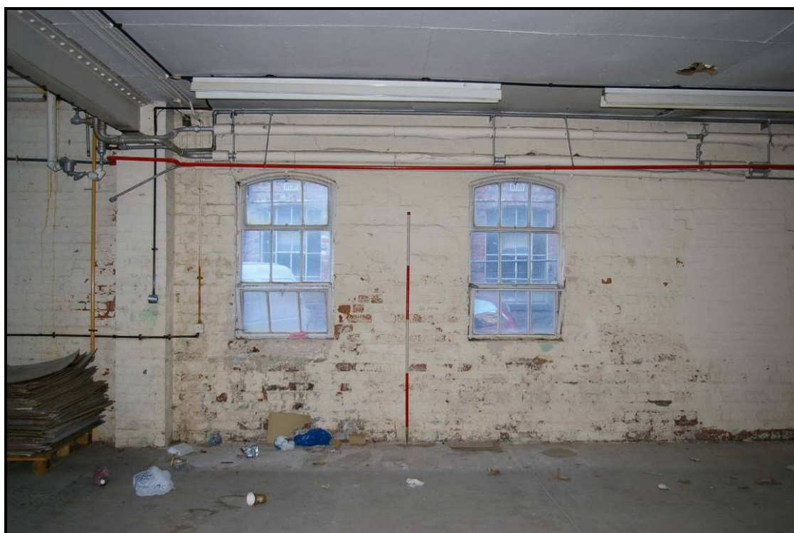
Figure 101: North wall of the ground floor of Building H with blocked doorway on the right
