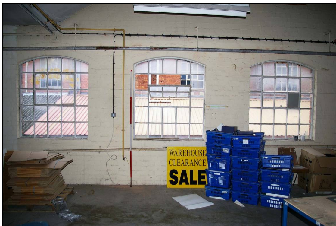
Figure 108: West wall on the northern half of the first floor of Building H
