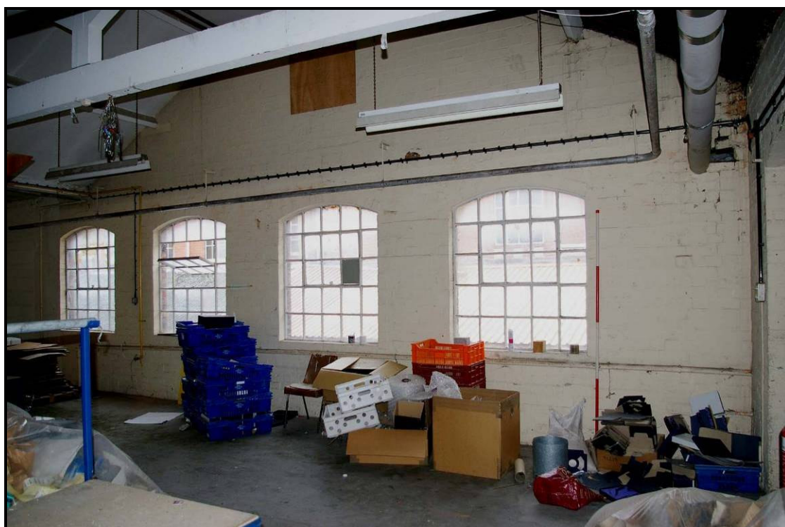
Figure 107: West wall on the northern half of the first floor of Building H
