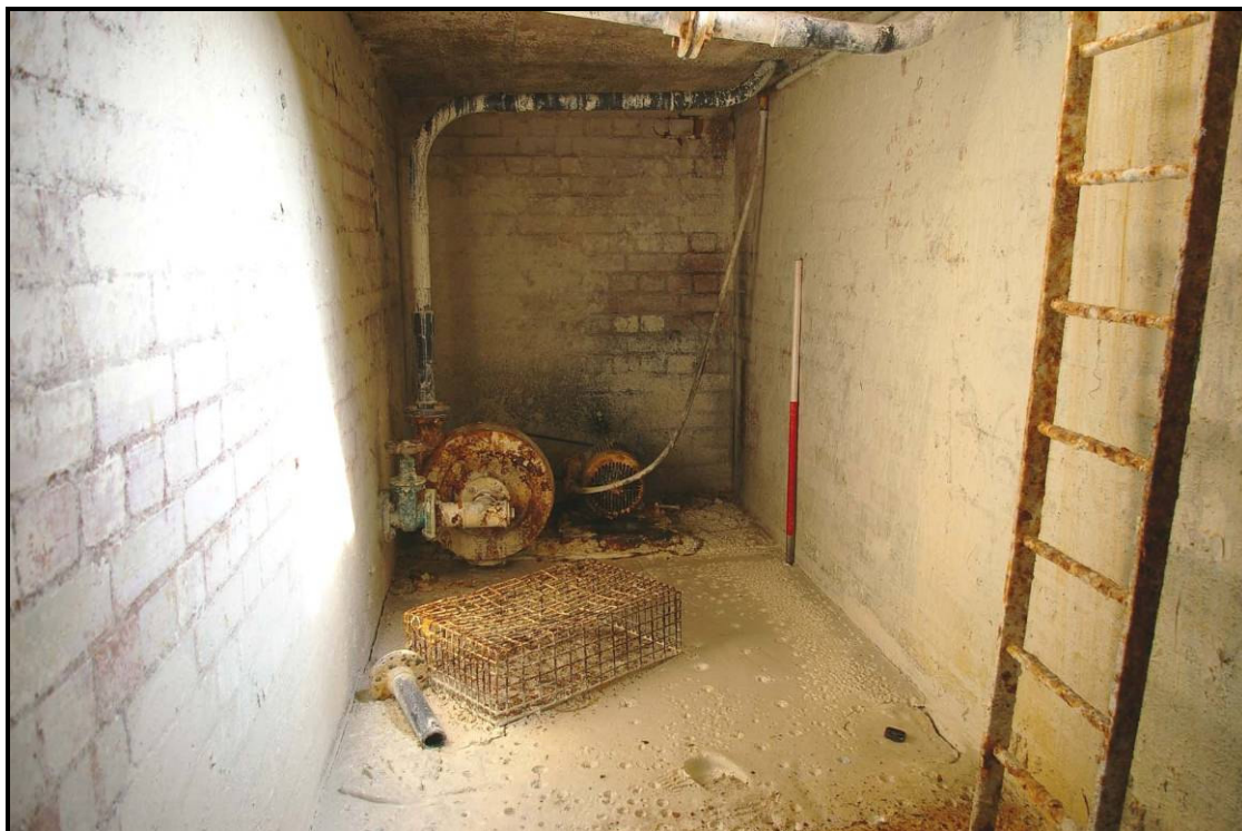
Figure 24: Underground tank, looking north
