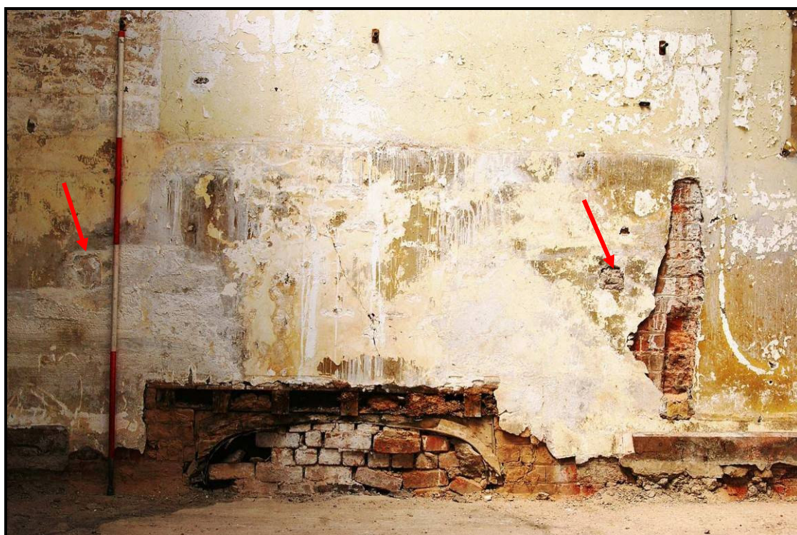
Figure 51: Archway and sockets for handrail (red arrows) of former staircase revealed after the dismantling of the raised platform on the west wall
