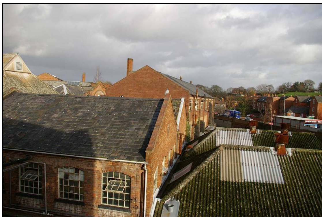
Figure 92: The east elevation of Building H butted by the hipped roof of Building I
