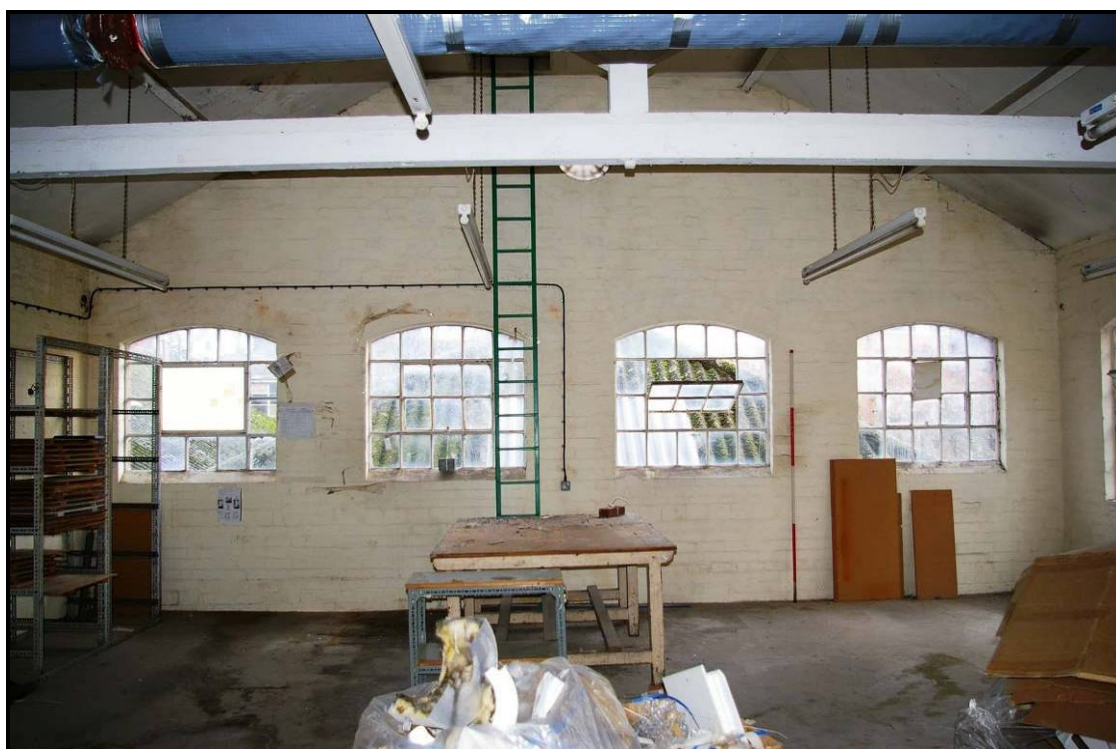
Figure 109: East wall on the northern half of the first floor of Building H
