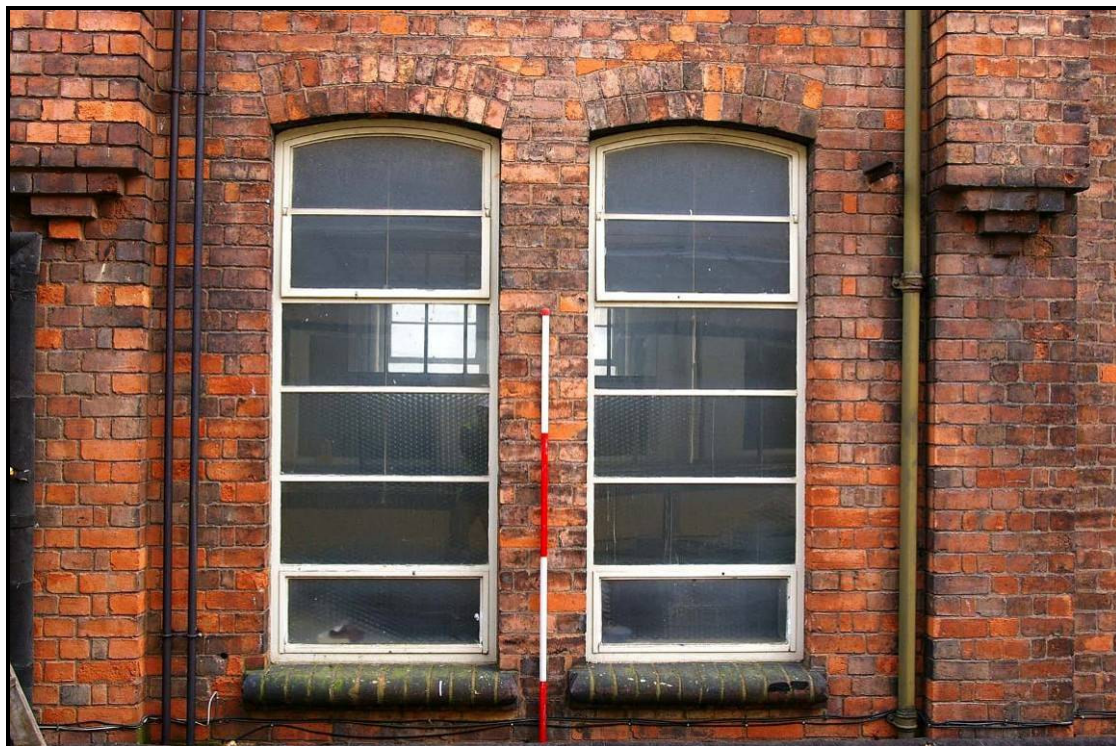
Figure 104: Detail of windows and corbelling on the first floor of Building R
