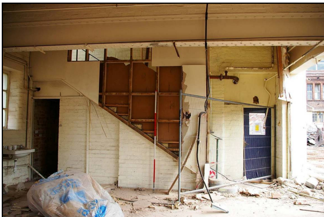
Figure 114: Ground floor of Building R showing inserted RSJ and stairwell, looking north
