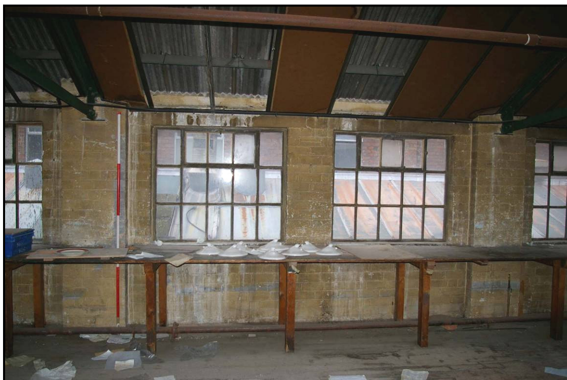
Figure 49: Windows on the south wall of the first floor of Building N
