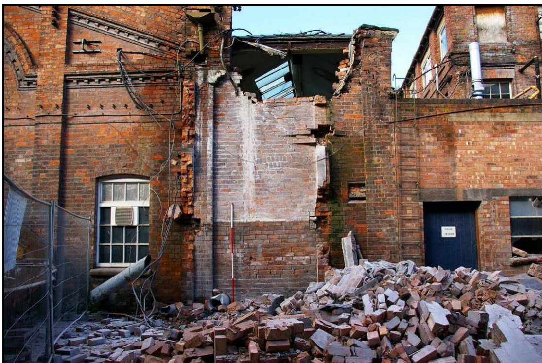
Figure 31: Blocked doorway of former lean-to of Building N revealed during its demolition
