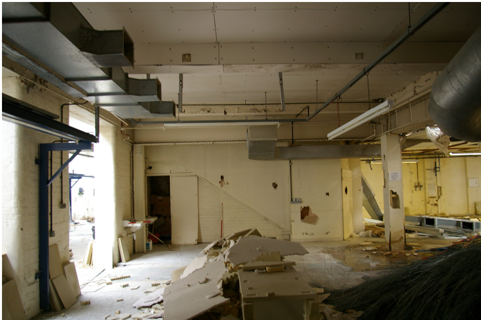
Figure 35: Looking north from inside the ground floor of Building R towards the boxed-in stairwell. On the left lies the knocked through wall to Building P and on the right lies Building S beyond the glazed area.
