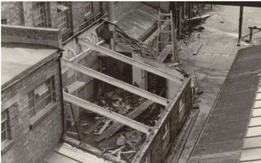
Figure 55: Building P under construction at the northern end (source: Worcester Porcelain Museum)
