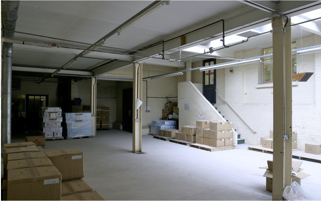
Figure 50: Building L, interior looking towards the exterior wall to Building J. The stairs that lead into Building J were originally exterior. Note the underpinning where the central wall has been removed.
