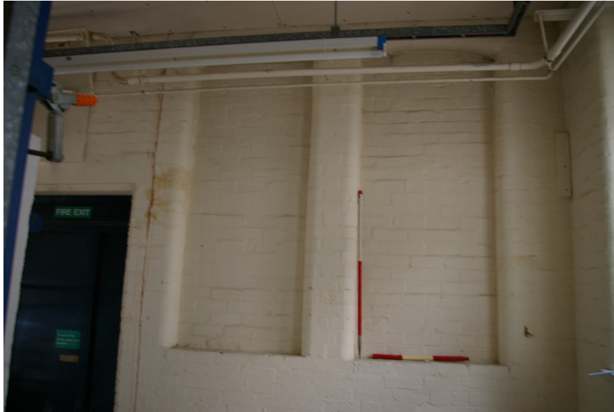
Figure 34: Building R, ground floor remains of east elevation from inside Building T
