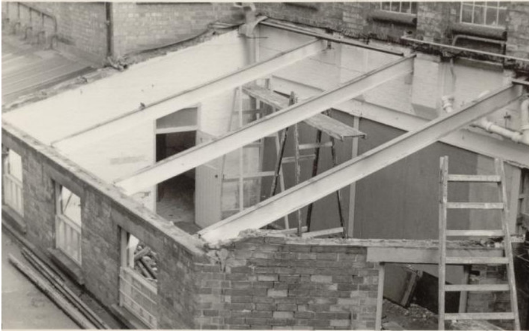
Figure 54: Building P under construction at the northern end (Building M lies behind with the lavatory block to the left. This lies on the site of the angled projection to M) (source: Worcester Porcelain Museum).
