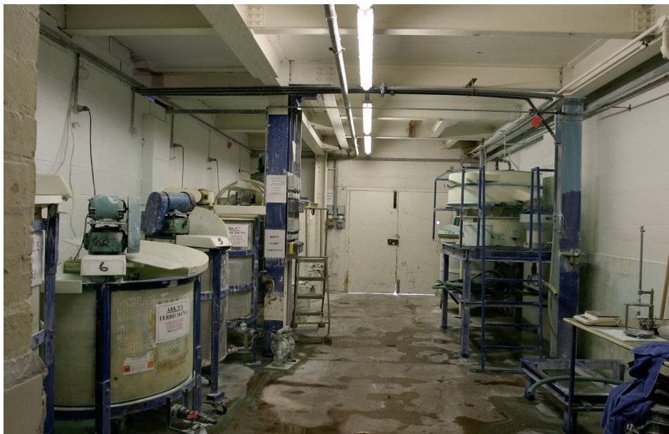
Figure 29: Building T, small ground floor room adjacent to east elevation of Building R
