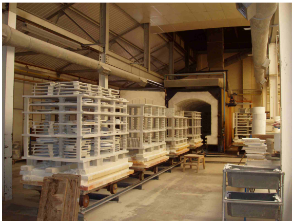
Figures 30, 31 and 32: China biscuit tunnel kilns on the first floor of Building T
