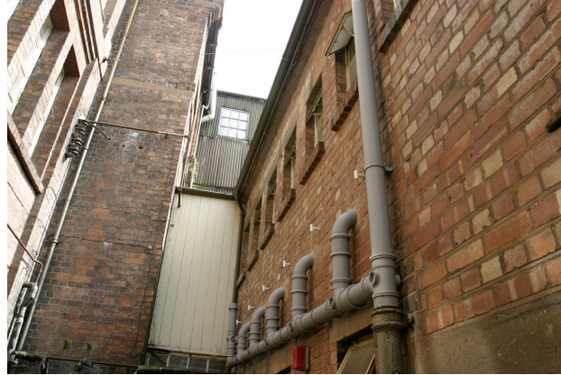
Figure 37: Building L1 (the lavatory block). This shows the windows and drainage to each cubicle in the female first floor part. Building J lies to the left with the over-bridges to Building M.
