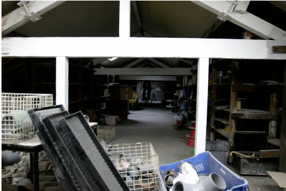
Figure 10: The adapted roof trusses of the 1875 building to make a central loft
