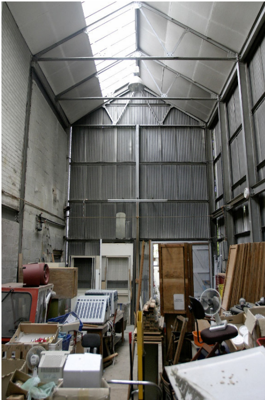
Figure 47: Interior of the cross-wing to Building Z. This was possible rebuilt in 1966 on the same footprint.
