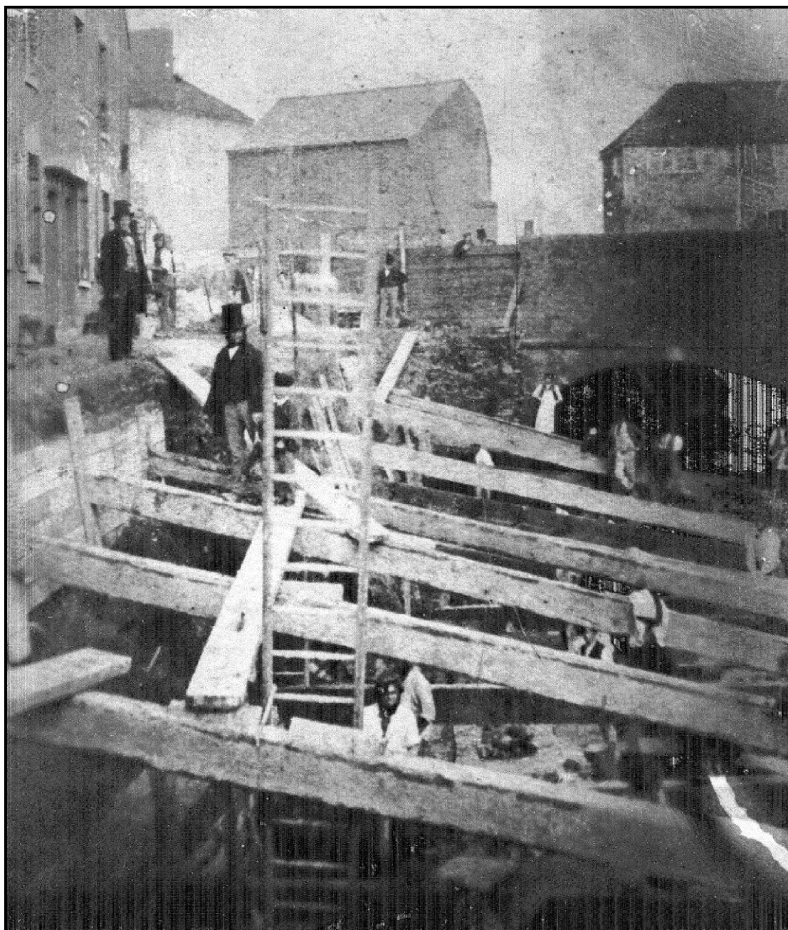
Figure 88: Repairing the canal wall during the late 19th century (courtesy of Worcester City Museum)
