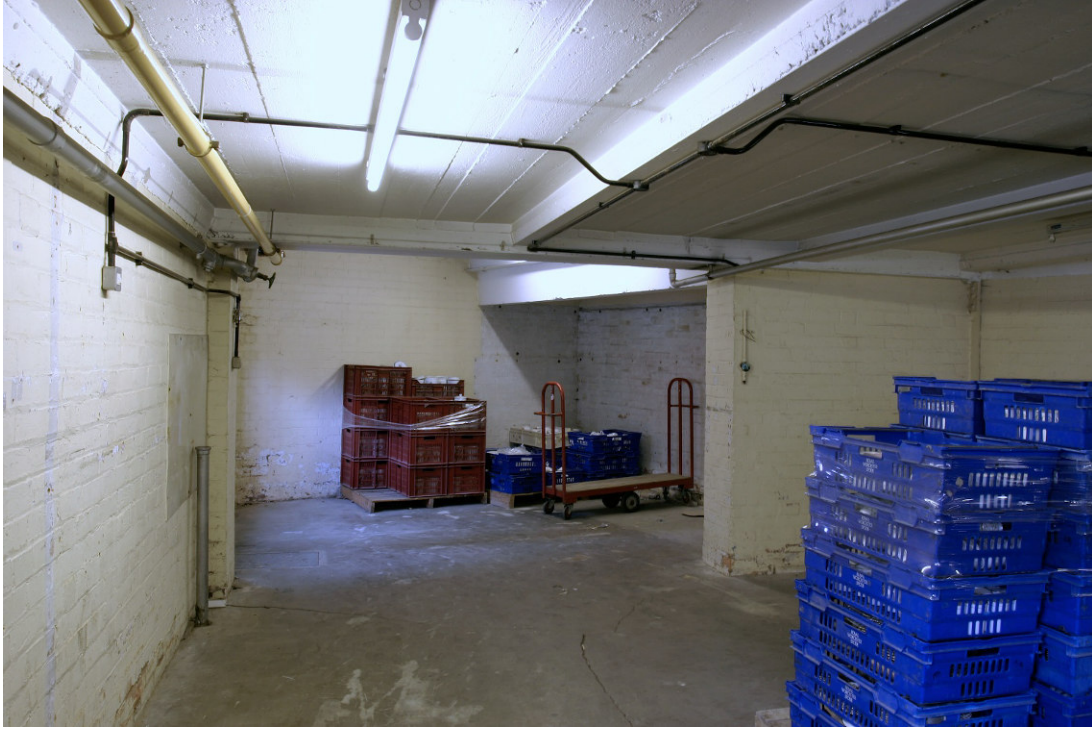
Figure 78: Building F. Ground floor supports at the narrow north end adjacent to Building C1.
