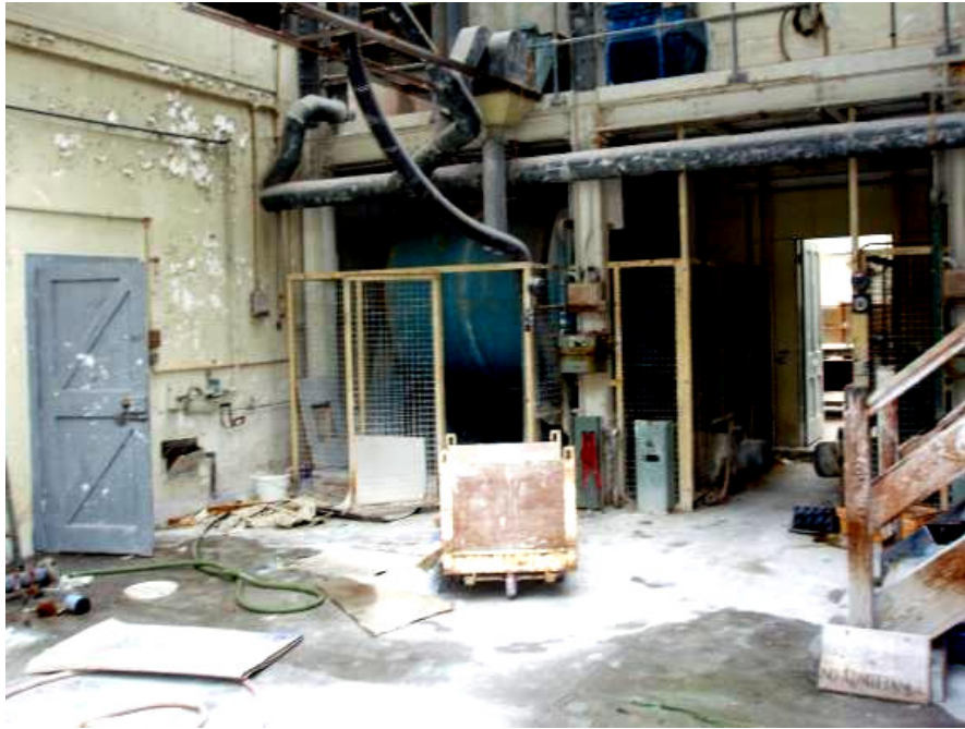
Figure 50: In Building A beneath the cross-wing looking north-east. The door on the left leads to the steel stairs. A rotary mill (mixer) lies to the left and the wooden stairs lead to the charging platform for the mills. Beyond through the door lie the laboratories.
