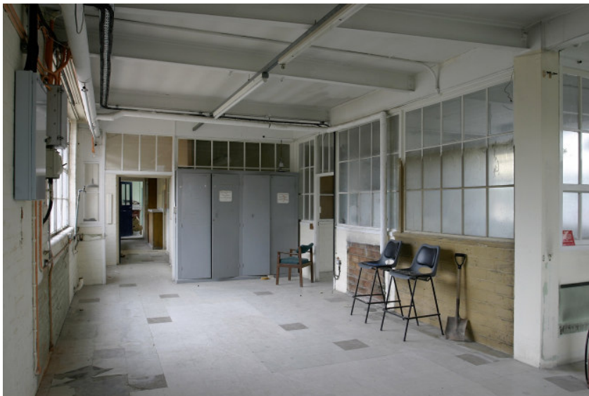
Figure 69: First floor of Building C1 looking towards Building B. The library lies to the left.
