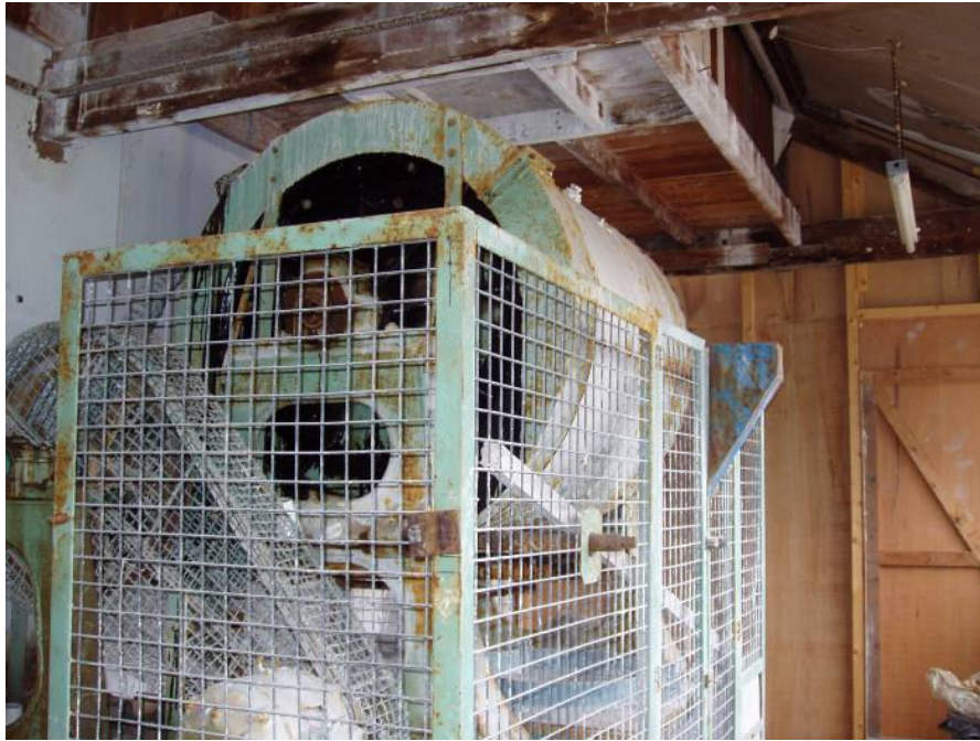
Figure 46: The rotary mixer in Building A2 by William Boulton
