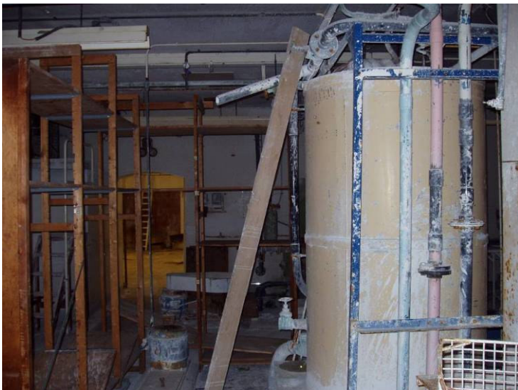
Figure 37: A holding tank in the Slip House
