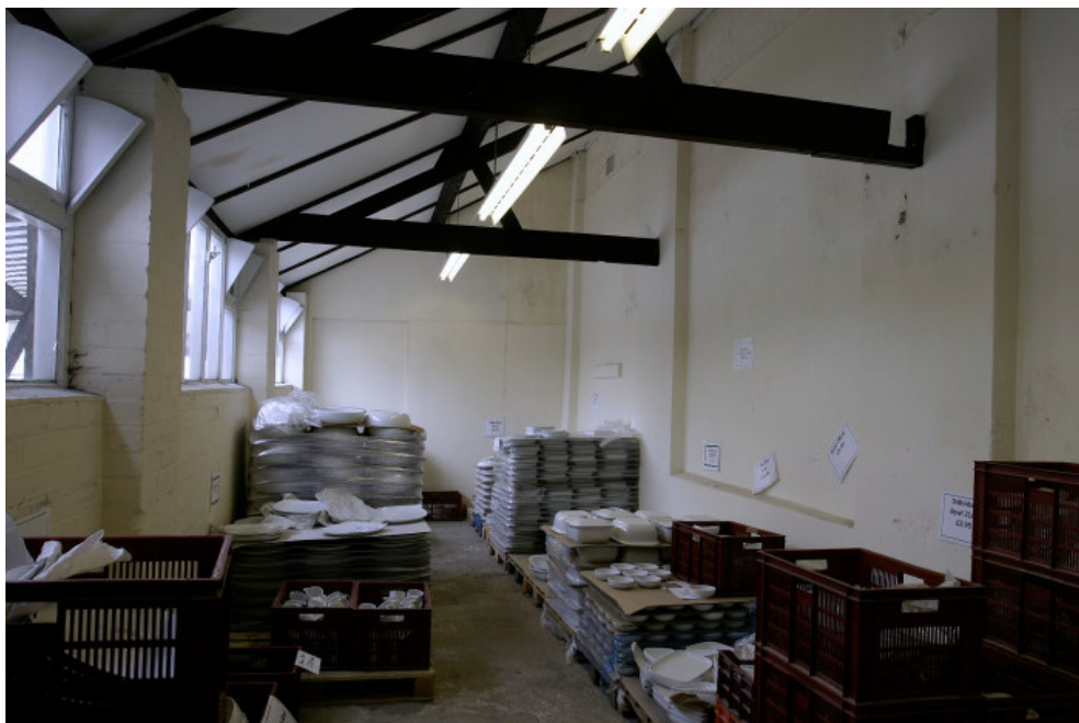
Figure 45: The lean-to Building A2. This can be dated to around 1940. The north wall of Building A is on the right. The roof trusses are made of wood.
