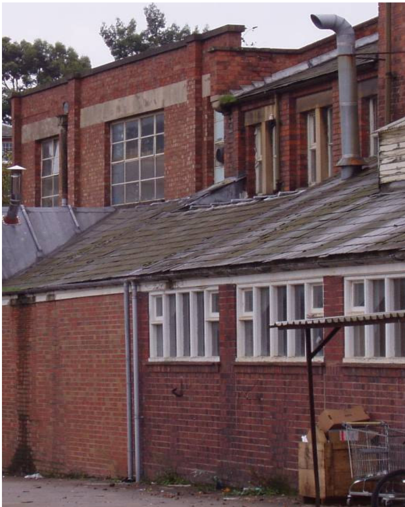
Figure 55: The north elevation of Building B lost amidst Buildings C1 (left), Building A2 (front) and Building A (right). Halfway up they turn into Building A but continue up to Building B.
