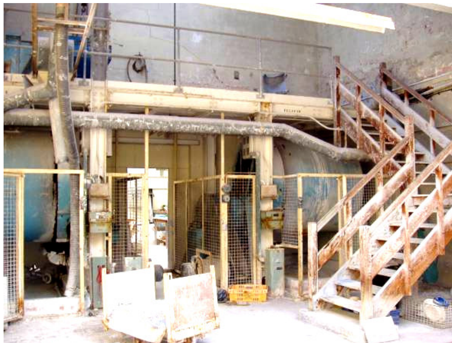
Figure 51: In Building A beneath the cross-wing looking south-east. A rotary mill (mixer) lies behind the wooden stairs which lead to the charging platform.
