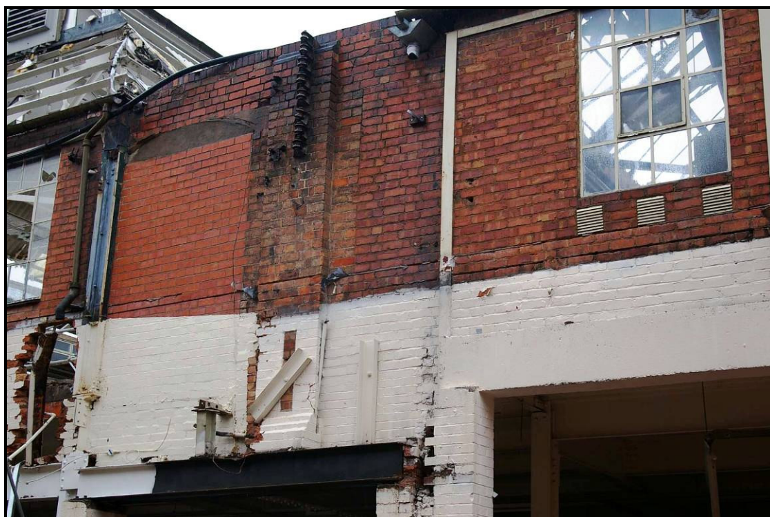
Figure 42: Detail of former pilaster and blocked opening of the earlier bridge on the east elevation
