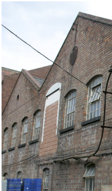
Figure 46: The original access to the bridge between Buildings H and G shown in the centre of the photograph
