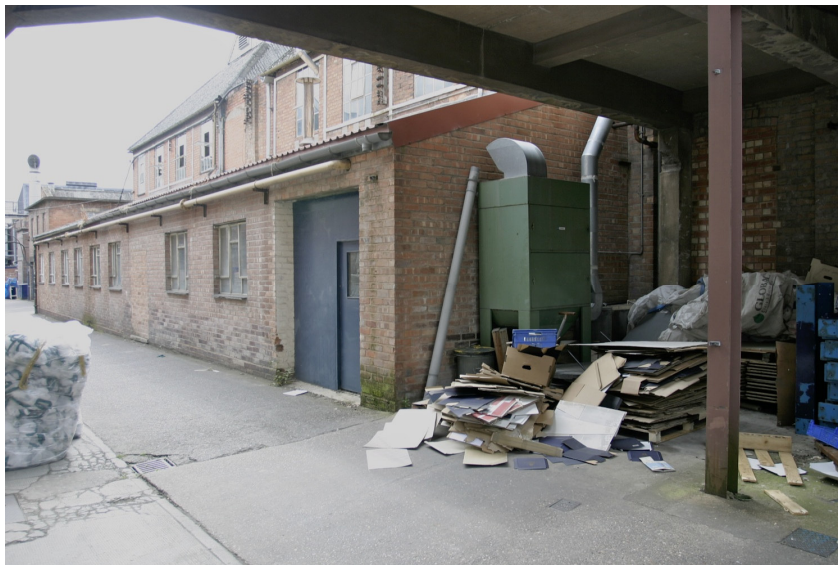
Figure 44: The post-1964 single-storey run in front of Building G from the north east. The building break where the line was extended beyond to the south can just be seen beyond the second window.
