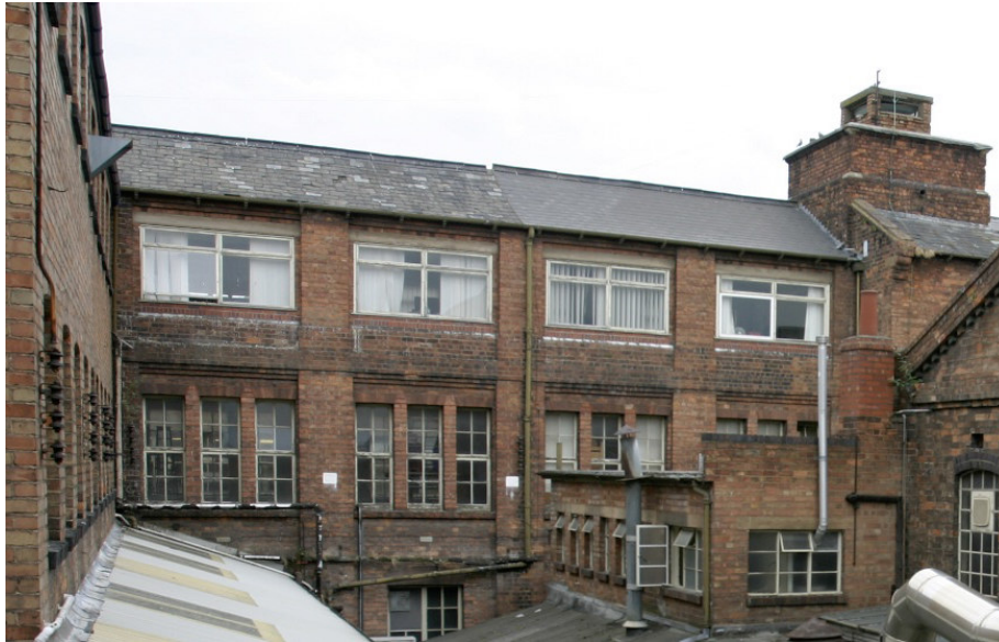
Figure 6: The rebuilt 1840s narrower part viewed from the south (centre). To the right is the eastern extension of 1854 to Building J with the truncated chimney above its west end. To the left is the 'New Wing' of 1874.
