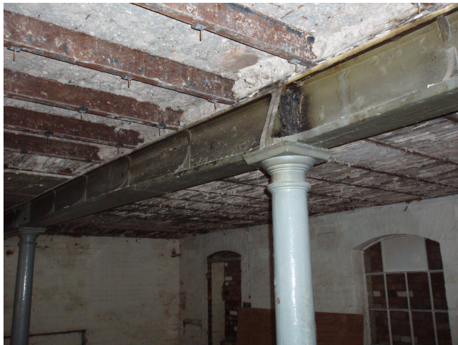
Figure 14: Modified Smirke beam used at Worcester (Building J) with cleared out Fox and Barrett fireproofing
