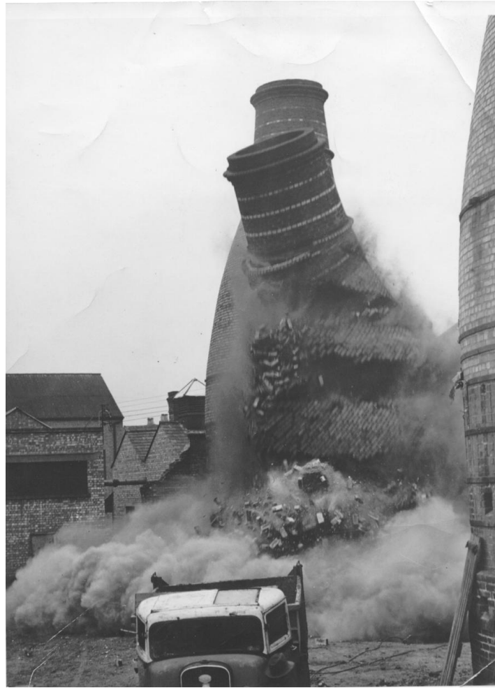
Figure 34: Demolition of the K3 kilns in the early 1950s (source: Worcester Porcelain Museum)
