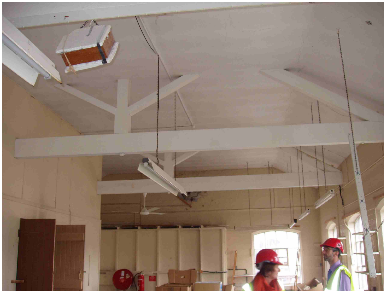
Figure 18: The top floor of Building K1 showing the roof trusses as designed by Sutton
