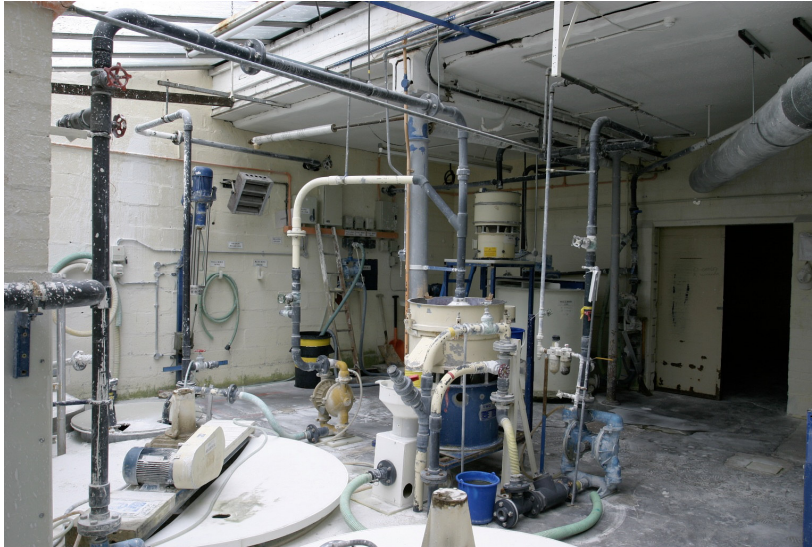
Figure 35: Slip machinery above the 1956 tanks in the north end of K3. After 1970 this extended into the Lady Caster Department which lay on the site of the former kilns – the division between the two is marked by the skylight to the left.
