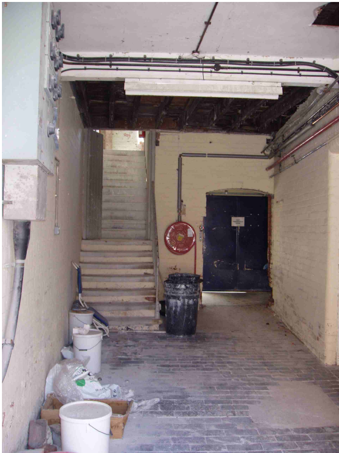
Figure 25: The odd-shaped space formed at the north end of K2 leading into K3
