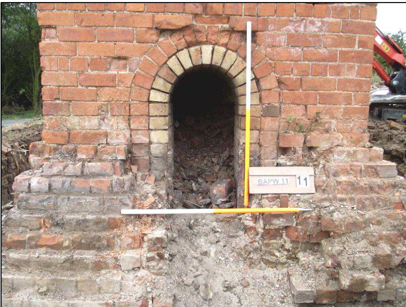
Plate 2: General view of the chimney opening and the foundation. North elevation, looking south
