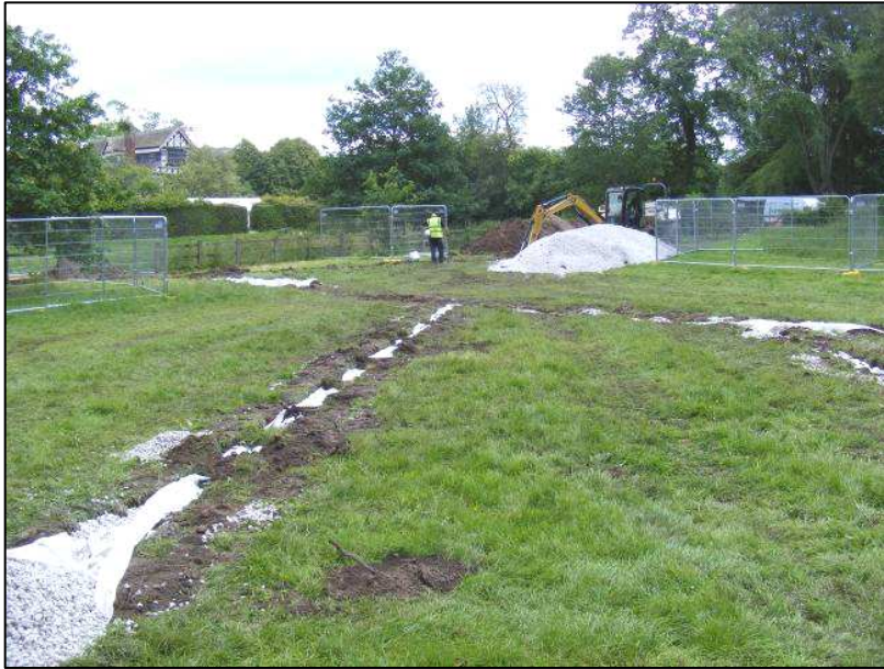
Plate 1: General shot across the groundworks looking south-east from the north-west corner of the site
