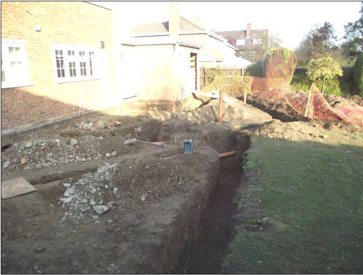
Plate 1: General view of the footings taken from the southern corner of the site, looking north
