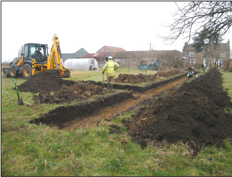
Plate 1: General view of the site during trial trenching. Taken from a position south-east of the excavation looking north-west with Trench 1 in the foreground and Trench 2 being machine excavated
