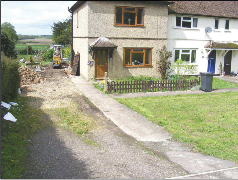
Plate 1: General view of the development area, looking west from the main road
