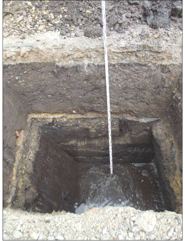
Plate 5: Test Pit 4 following excavation, showing east facing section and looking west. Measuring staff to top of trench is 4m high
