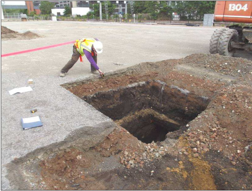
Plate 1: Test Pit 1 under machine excavation. Showing temporary fall arrestor system in use and using laser measuring device. Looking north-west
