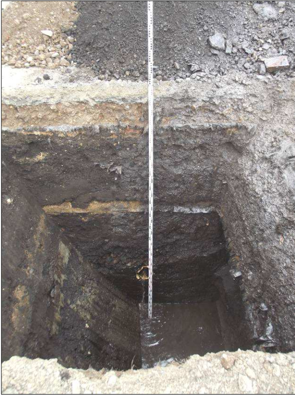
Plate 4: Test Pit 3 following excavation, showing east facing section and looking west. Measuring staff to top of trench is 4m high
