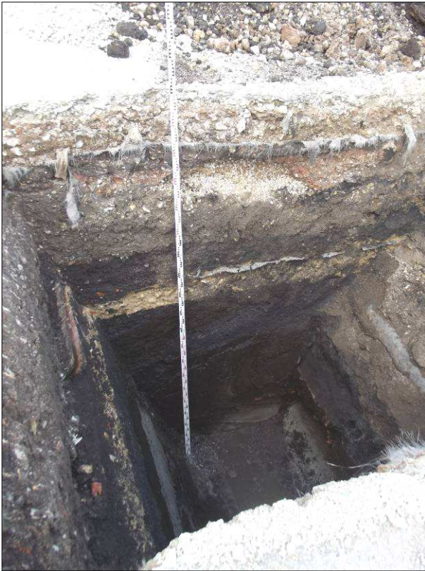
Plate 2: Test Pit 1 following excavation, showing east facing section and looking west-north-west. Measuring staff to top of trench is 4m high
