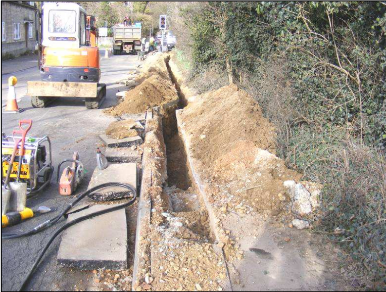
Plate 1: General working shot showing electric cable trench along High Dike and Ermine Street, looking northeast
