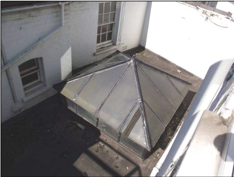
Plate 7 (Shot 8): View of skylight in ground floor flat roof extension, looking south-west
