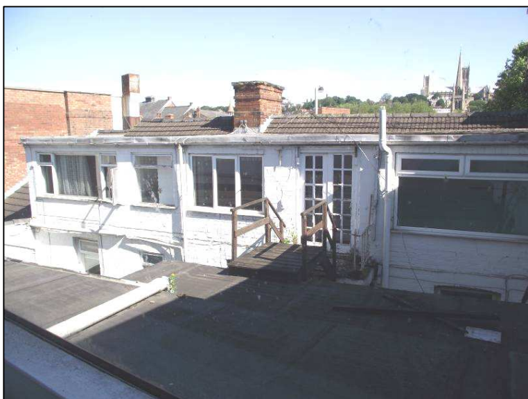
Plate 6 (Shot 9): South elevation of range fronting onto Norman Street, taken from second floor, looking north-west. Note intervening flat roof extensions
