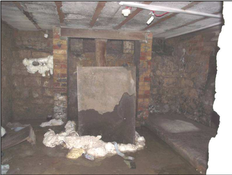
Plate 14 (Shot 66): Possible former boiler room at west end of basement below the kitchen. Also note the earlier limestone walling, looking west-northwest.
