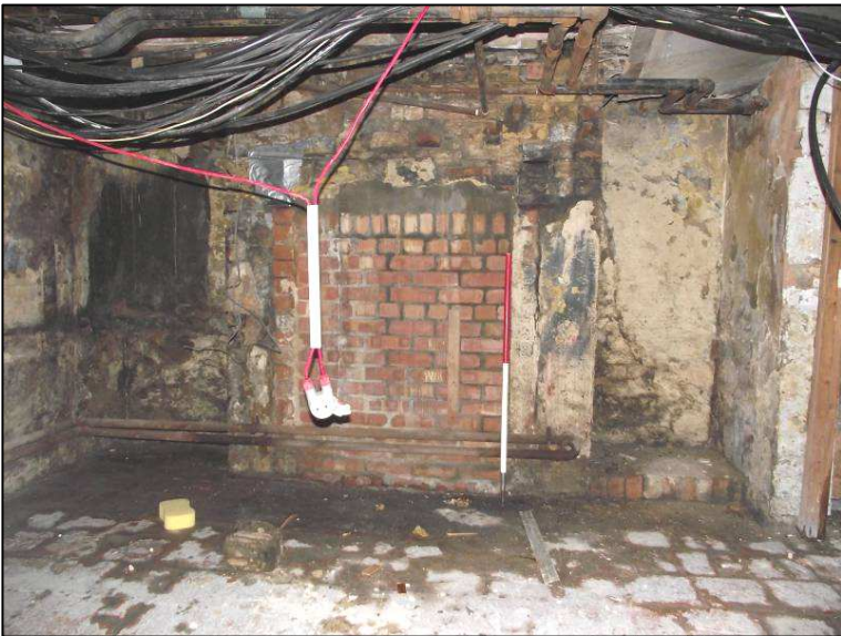
Plate 8 (Shot 62): Bricked up fireplace and quarry tile floor in the basement, looking east-southeast. Scale is 1m
