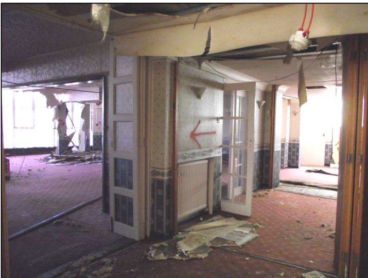
Plate 17 (Shot 39): Dining rooms in northeast portion of ground floor, looking east- northeast
