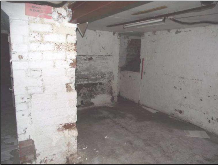
Plate 13 (Shot 57): Storage area with coal chute in the corner, looking north-west. Scale is 1m
