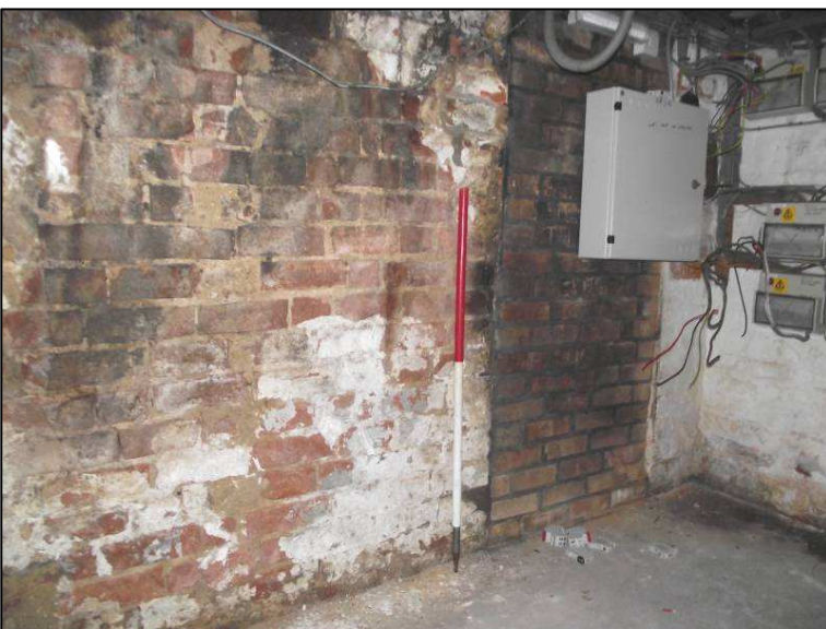
Plate 12 (Shot 61): Bricked up opening between easternmost store rooms, looking south-west. Scale is 1m
