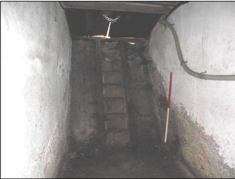
Plate 10 (Shot 46): Basement access to beer cellar from St. Mary's Street, looking south-southwest. Scale is 1m
