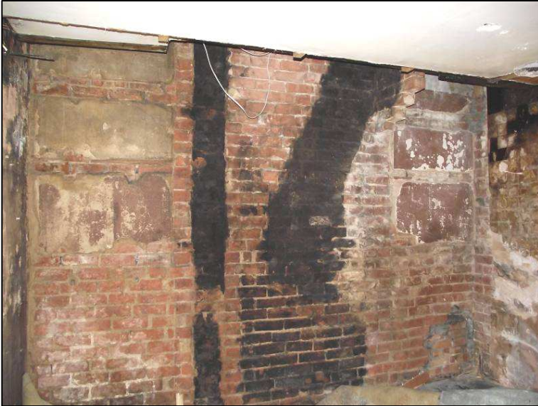
Plate 16 (Shot 42): View of location of former chimney breast on ground floor, (situated above fireplace in Plate 11), looking east-southeast.
