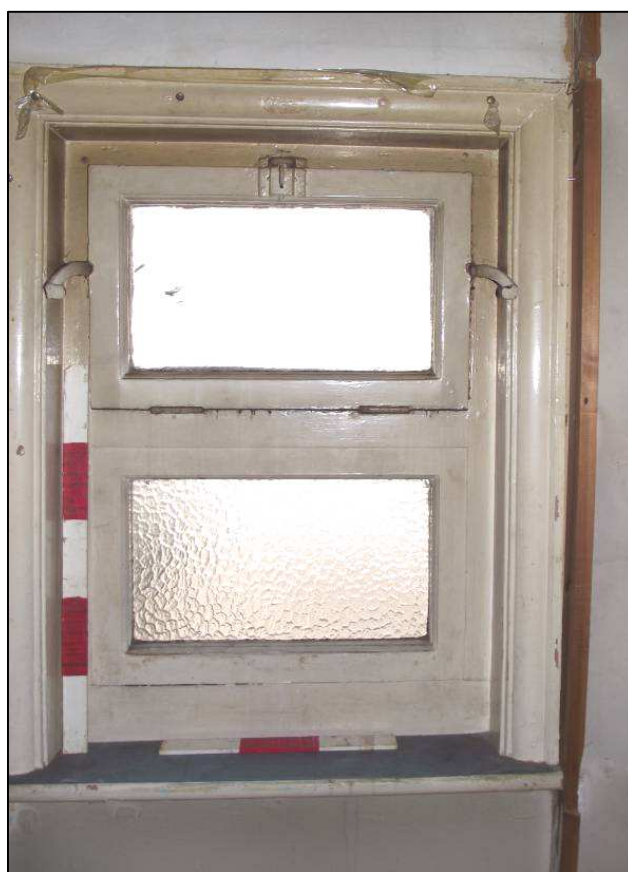
Plate 21 (Shot 25): Small hopper window in storage area on first floor, looking north-northeast. Scales are 0.5m and 0.3m
