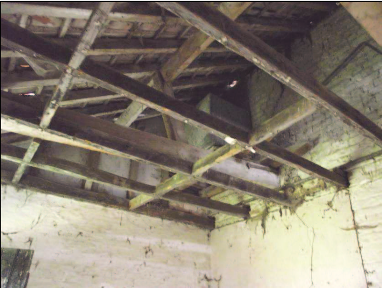
Plate 8 (Shot 34): Floor joists and water tank in Room 1 of Barn 1, looking north
