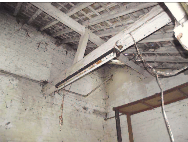
Plate 9 (Shot 37): Roof structure in Room 2 of Barn 1 showing metal water pipe. Looking southeast
