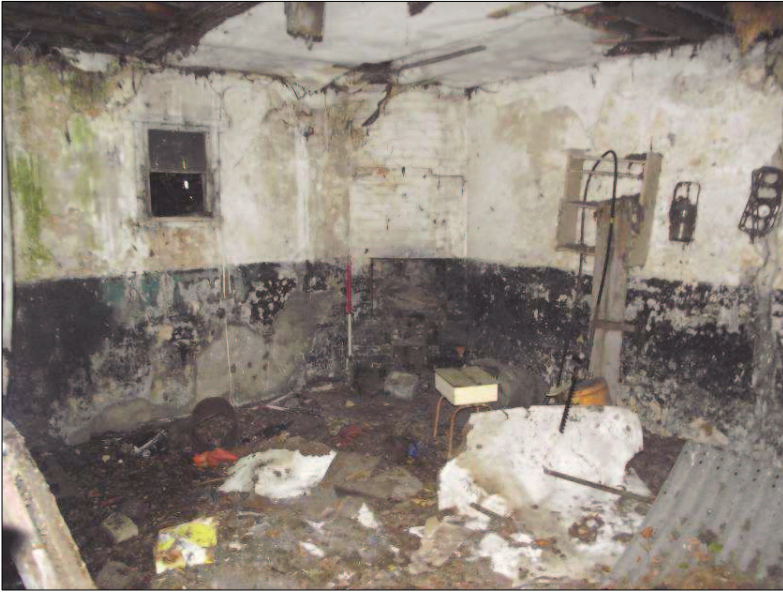
Plate 16 (Shot 27): Tack room/crew room at west end of Barn 2, looking southwest towards fireplace. Scale is 1m
