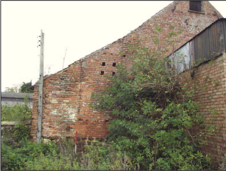
Plate 4 (Shot 8): South elevation of Barn 1 showing possible ventilation holes and bricked up opening, looking north. Scale is 1m
