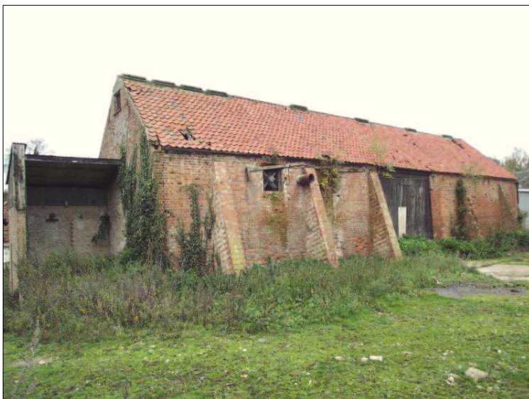
Plate 2 (Shot 5): South end of Barn 1, looking west-northwest, showing area of repair and extension to south end of the barn. Also note the ventilation fan and outlet pipe in this elevation
