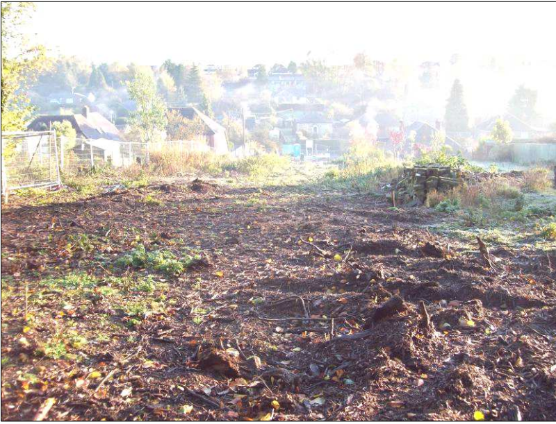
Plate 1: General site shot before groundworks, looking east-northeast from the west end of the site
