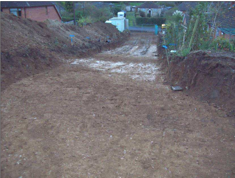
Plate 2: General view of access road strip along southern half of site, looking east-northeast. Note extent of ground reduction shown by section to right of shot
