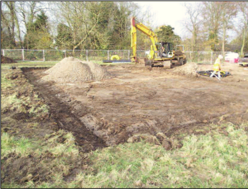
Plate 1: General site shot, looking north
