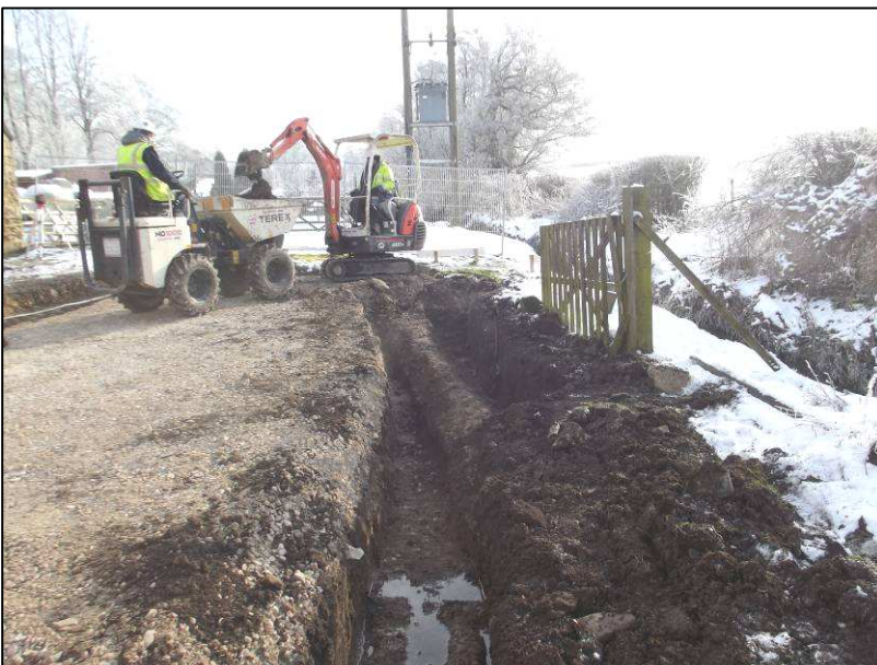
Plate 3: Excavation of foundation trenches, showing the modern sewer pipe (Figure 3). Looking southeast.
