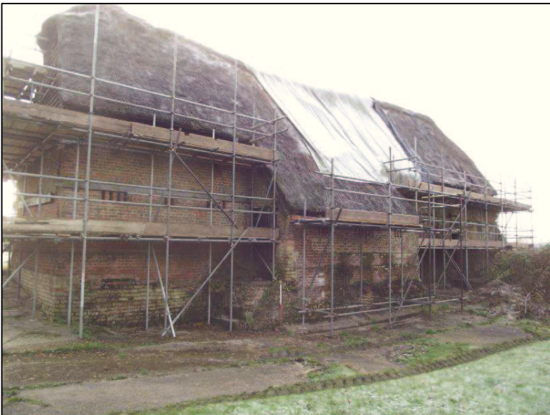
Plate 5 (Shot 23): North elevation of the barn with outshut, looking southwest. Scale is 1m
