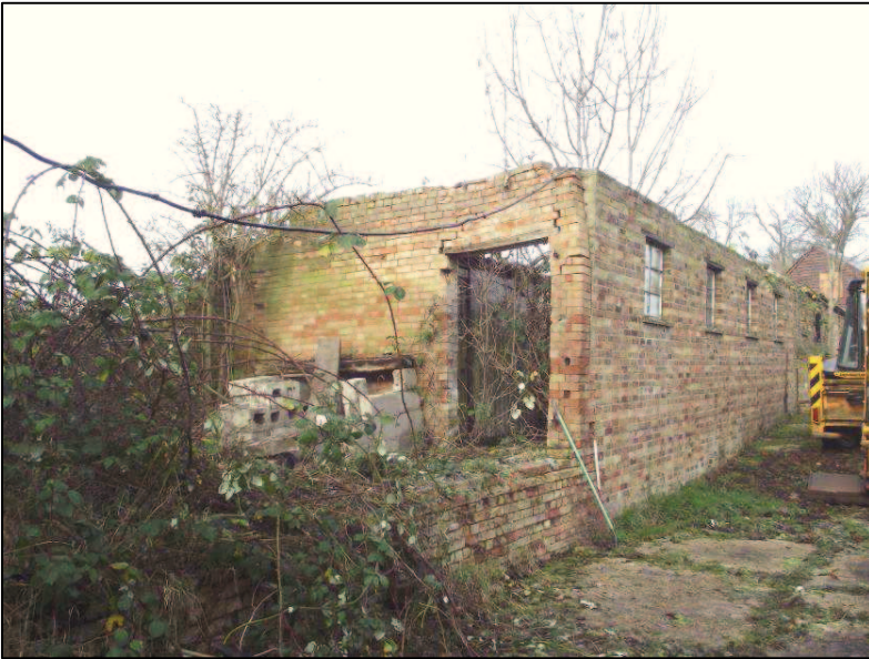
Plate 17 (Shot 27): North elevation of Outbuilding 1 and east elevation of Outbuilding 2, looking northwest. Scale is 1m
