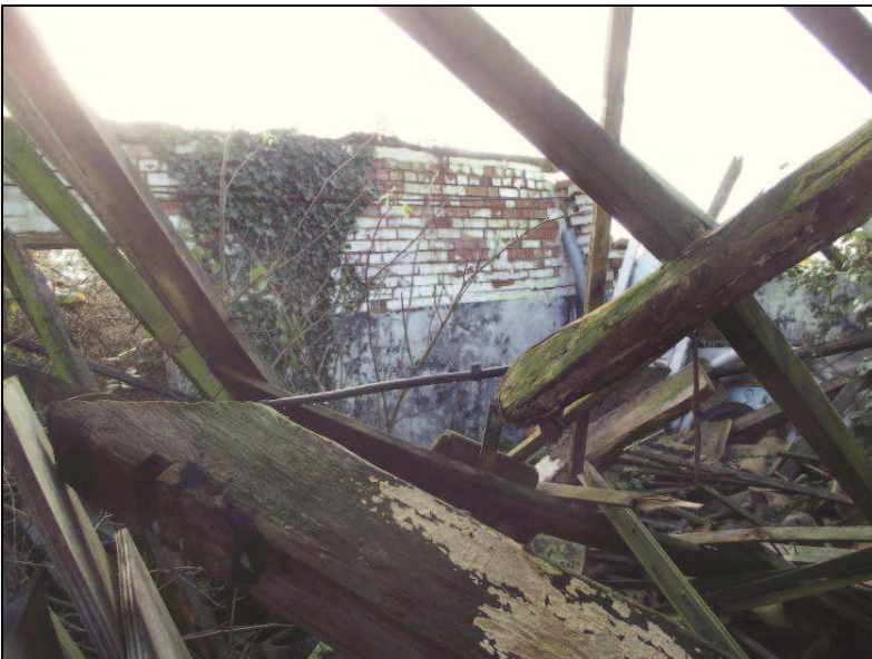
Plate 21 (Shot 36): Interior view of demolished/ collapsed Outbuilding 3 looking southwest
