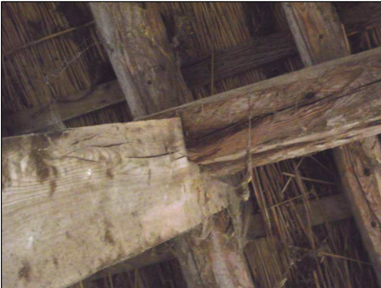
Plate 14 (Shot 19): Detailed shot of trenced purlin, looking up and to the south
