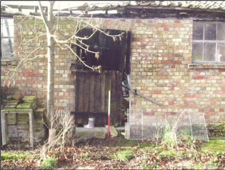
Plate 20 (Shot 31): East elevation of Outbuilding 3, showing stable door, looking west. Scale is 1m
