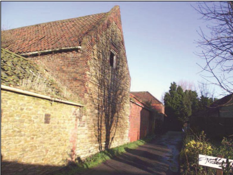
Plate 14 (Shot 1): Southeast elevation of B2 and B3, looking north. Scale is 2m
