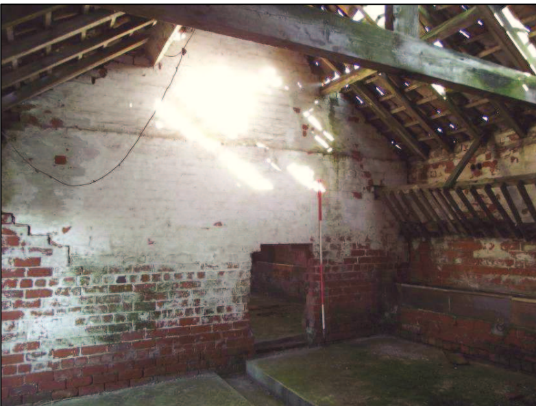
Plate 21 (Shot 24): Interior view of B3.3 with opening formed to B.3.4, looking northeast. Scale is 2m
