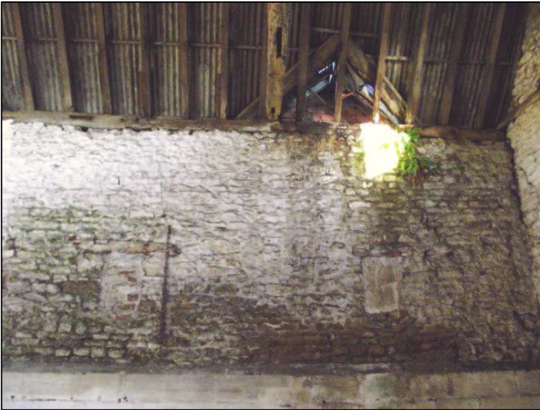
Plate 16 (Shot 16): Blocked up openings on northeast elevation, also showing the adjoining B3, looking northeast
