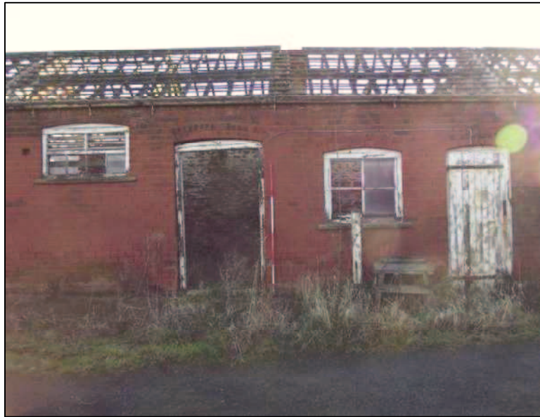
Plate 4 (Shot 5): Representative shot of B1 openings and windows, looking east-southeast. Scale is 2m
