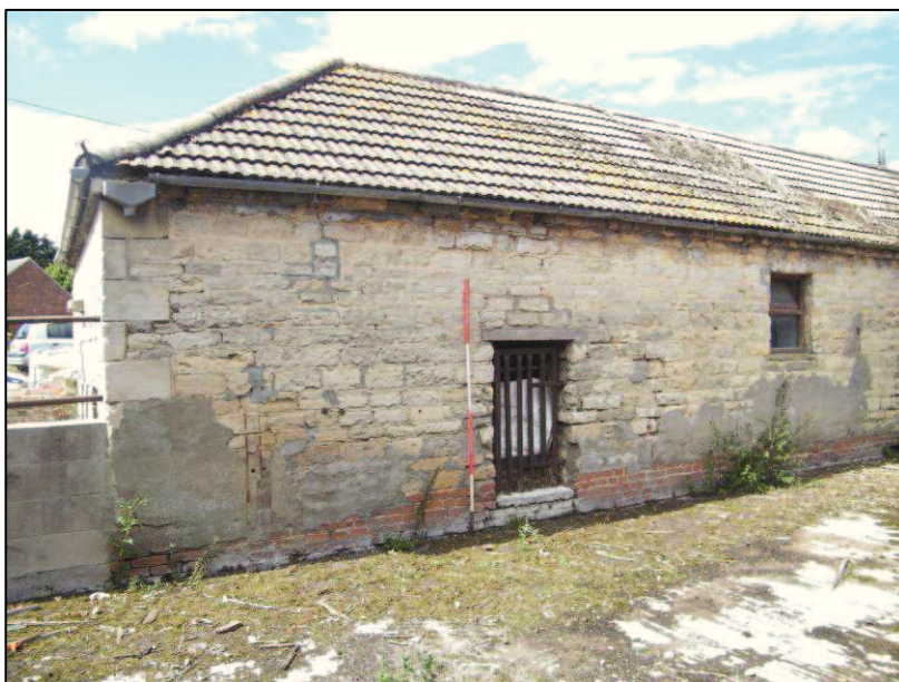
Plate 28 (Shot 52): Southern end of on the east elevation of Building C, looking west northwest, looking north. Scale is 2m
