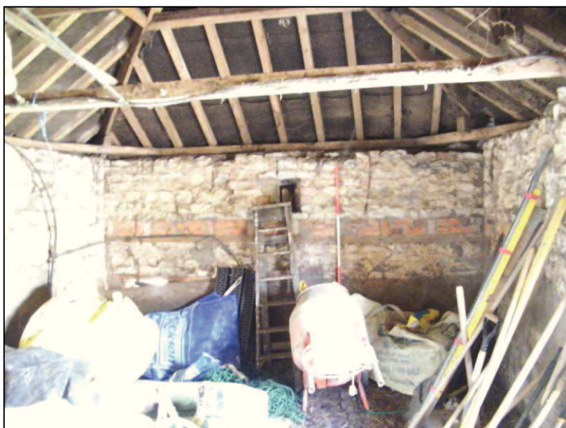
Plate 33 (Shot 61): Interior view of southern block of Building C, looking south-southwest. Scale is 2m
