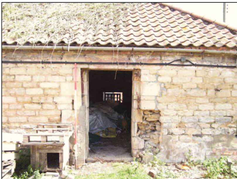
Plate 31 (Shot 59): South end of west elevation of Building C showing exposed rubble core, looking east northeast. Scale is 2m
