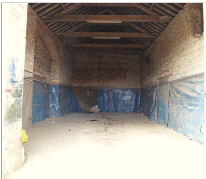
Plate 9 (Shot 16): Interior view of the threshing barn in Building A, looking west-northwest. Scale is 2m
