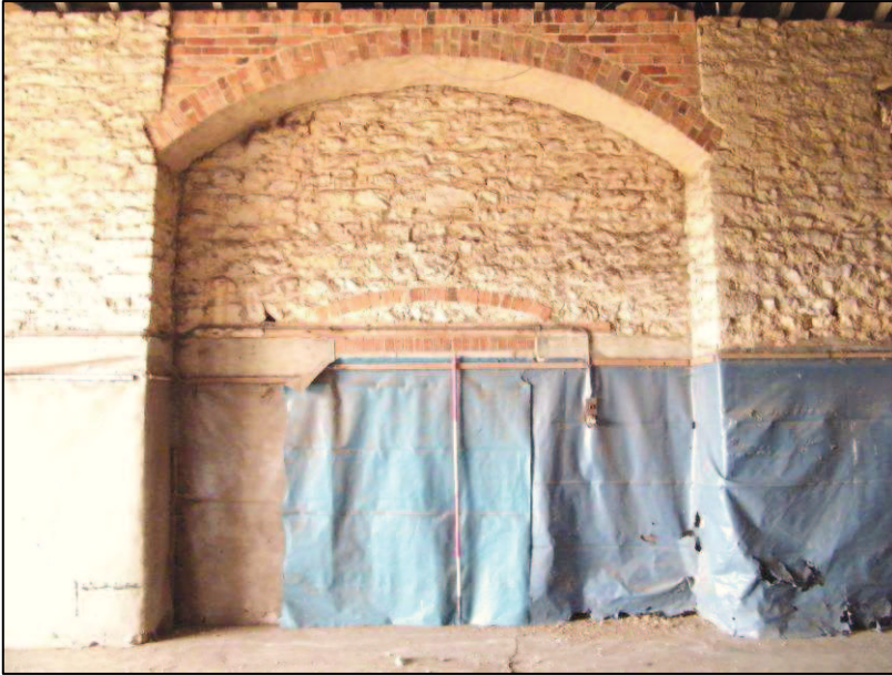
Plate 10 (Shot 18): Detail shot of the brick arch on the southern elevation in the threshing barn, looking south southwest. Scale is 2m
