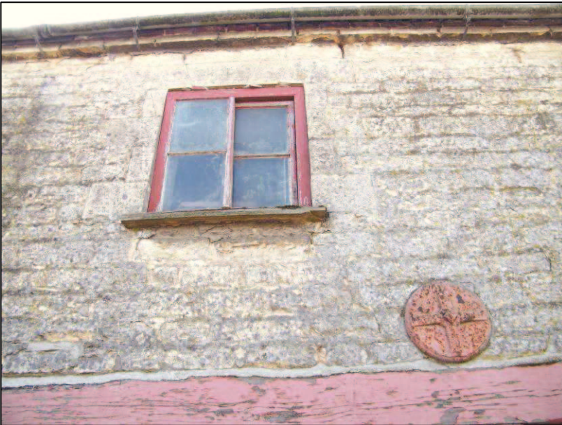
Plate 5 (Shot 6): Representative shot of first floor window and tie plate on north elevation of Building A.
