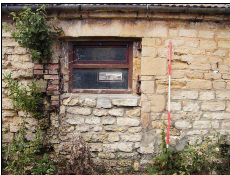
Plate 27 (Shot 50): Representative shot of a door converted into a window, east elevation of Building C, looking west-northwest. Scale is 2m
