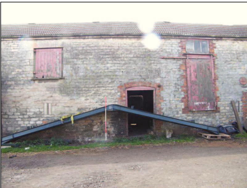
Plate 3 (Shot 4): Mid section of the north elevation of Building A showing brick dressings around openings, looking south-southwest. Scale is 2m
