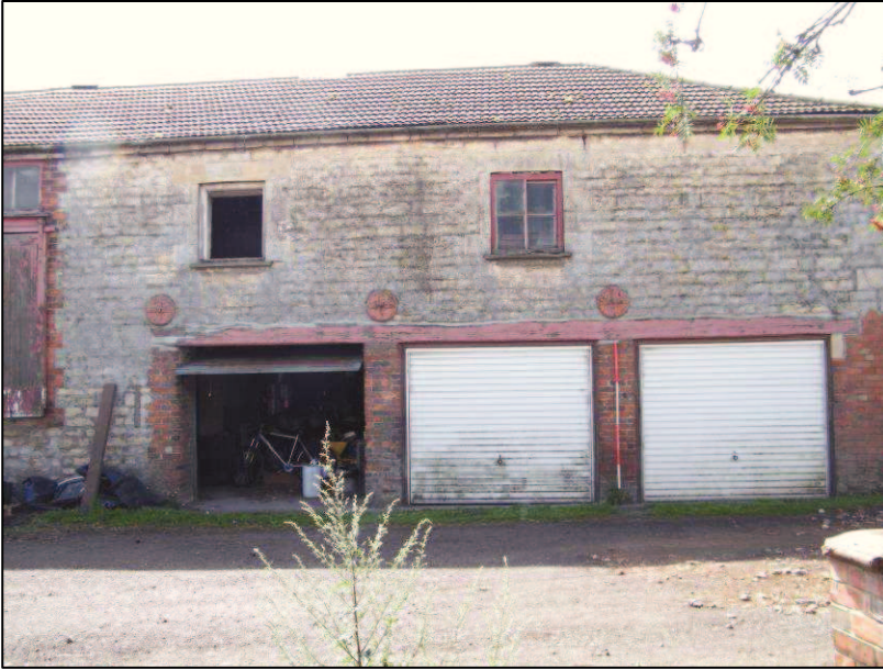
Plate 4 (Shot 5): West end of north elevation of Building A, showing garage doors. Scale is 2m
