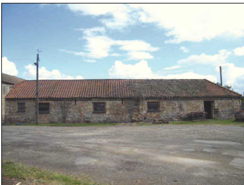
Plate 30 (Shot 55): West elevation of Building C, looking east northeast. Scale is 2m
