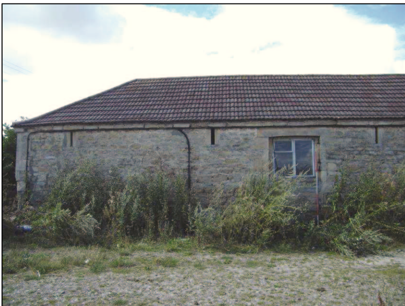
Plate 19 (Shot 37): East elevation of Building B showing blocked up door, looking west-northwest
