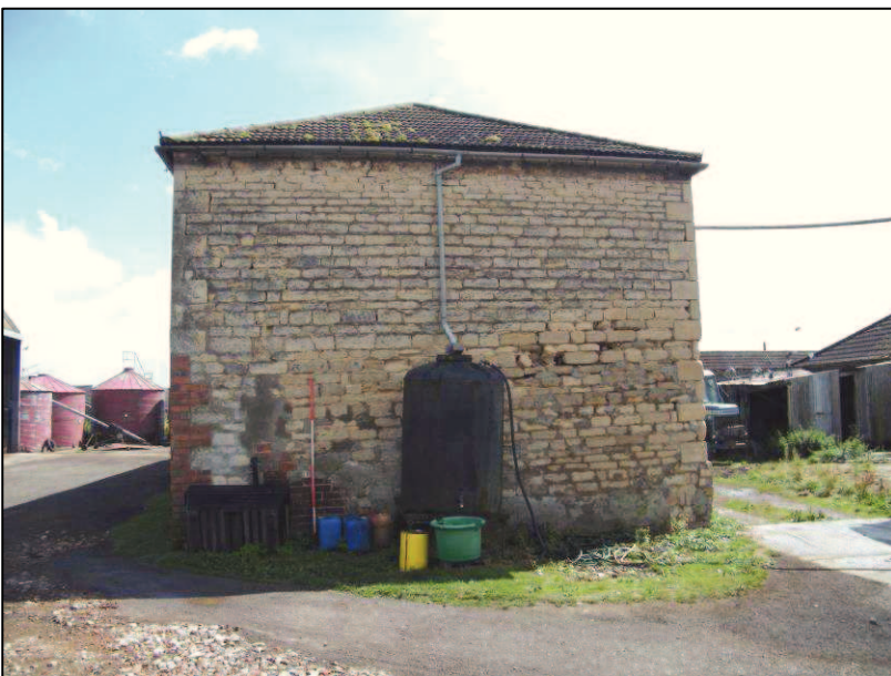
Plate 6 (Shot 10): West elevation of Building A, looking east southeast. Scale is 2m
