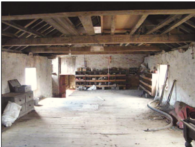
Plate 13 (Shot 25): Loft above west end of Building A, looking east-southeast. Scale is 2m
