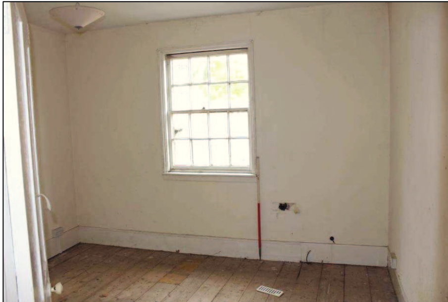
Plate 25 (Shot 22): First floor living space in the extension, looking west, 1m scale
