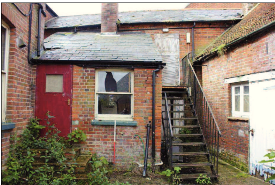
Plate 27 (Shot 100): In the background is the northeast elevation of the function room, in the foreground is a small kitchen extension, looking southwest, 1m scale
