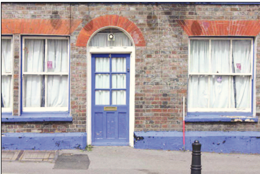
Plate 3 (Shot 120): Representative shot of ground floor doors and windows, looking northwest. 1m scale
