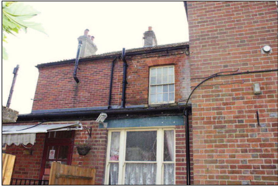
Plate 7 (Shot 110): Northwest elevation showing later rusticated brick repair, looking east
