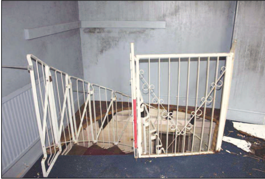
Plate 31 (shot 63). Spiral staircase between first floor and ground floor, looking northeast, 1m scale
