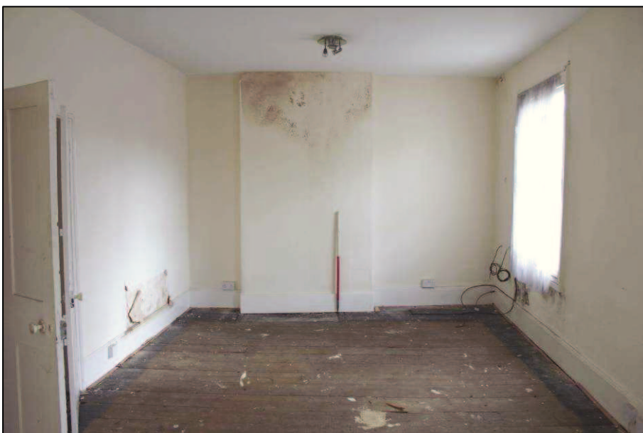
Plate 15 (Shot 26): Living space on first floor looking at blocked up fireplace on the northeast partition wall, 1m scale
