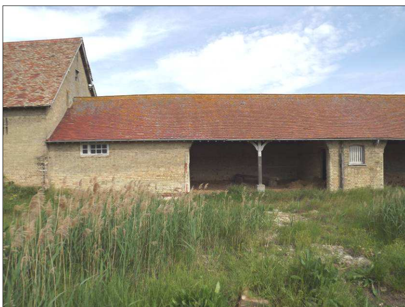
Plate 5 (Shot 3): Building B south elevation showing B1 –B3, looking north-northwest. 2m scale
