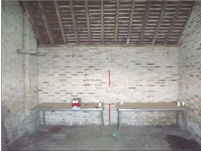
Plate 6 (Shot 55): B1 interior, looking north-northwest. Note former floor joists in wall to left of shot. 2m scale
