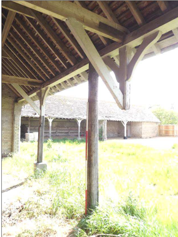
Plate 11 (Shot 43): Detail of cut off roof support and replacement post, looking southeast. 2m scale
