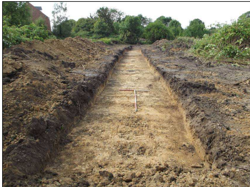
Plate 3: Trench 9 looking southwest. Scales are 1m. The modern service is located at the far end of the trench
