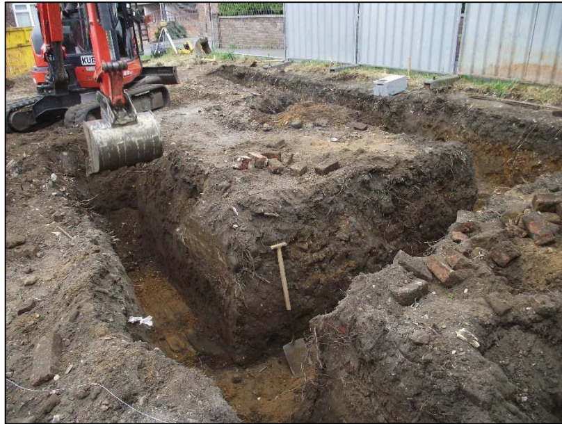
Plate 3: General view of structure 009 with north-south footings centre right of photograph, looking northeast
