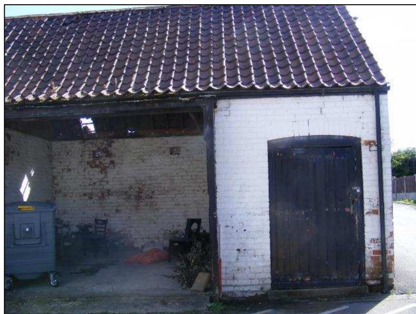
Plate 14 (shot 7): North facing elevation of east-west aligned range of stable block. 1m scale
