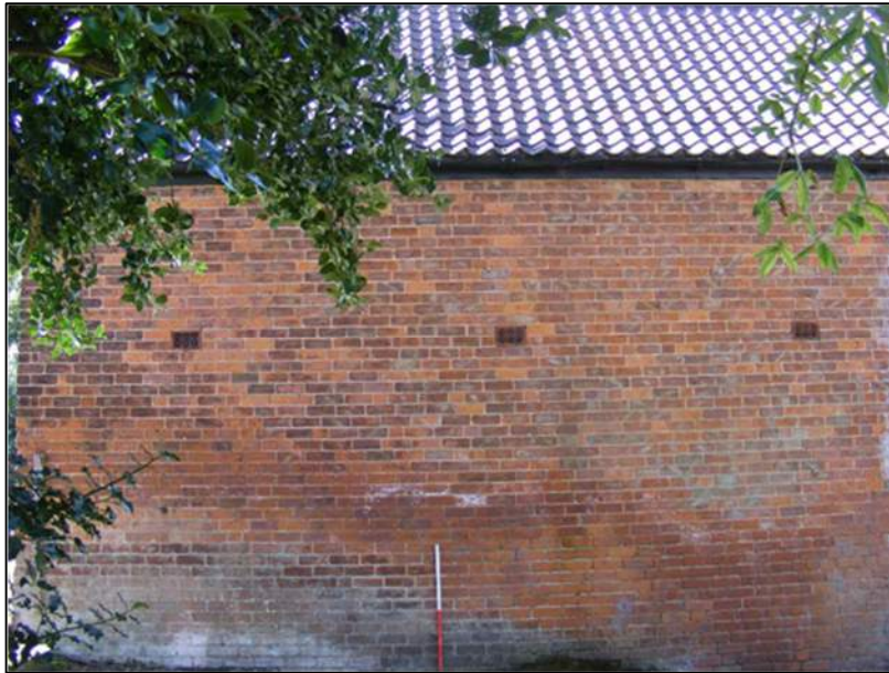
Plate 8 (shot 3): East facing elevation of north-south aligned range of stable block, southern end. 1m scale
