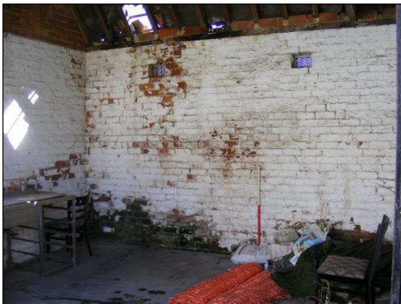
Plate 18 (shot 10): Interior of Room B, east-west aligned range of stable block. 1m scale
