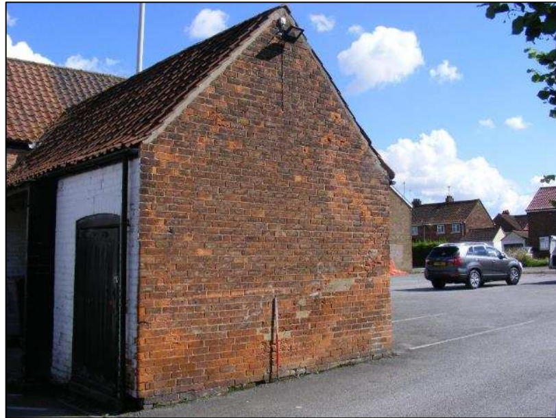
Plate 13 (shot 6): West facing elevation of western gable end of east-west aligned range of stable block. 1m scale
