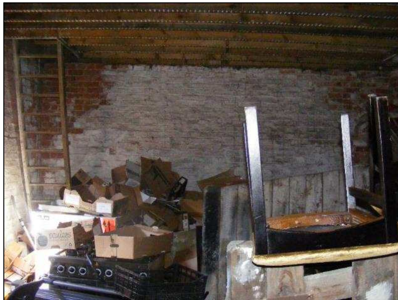
Plate 17 (shot 13): Interior of north-south aligned range, looking north. Timber stall division visible on left hand side. Access ladder to hayloft on right hand side.
