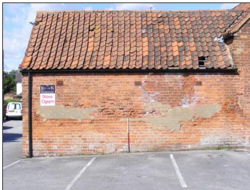
Plate 12 (shot 1): South facing elevation of east-west aligned range of stable block. 1m scale
