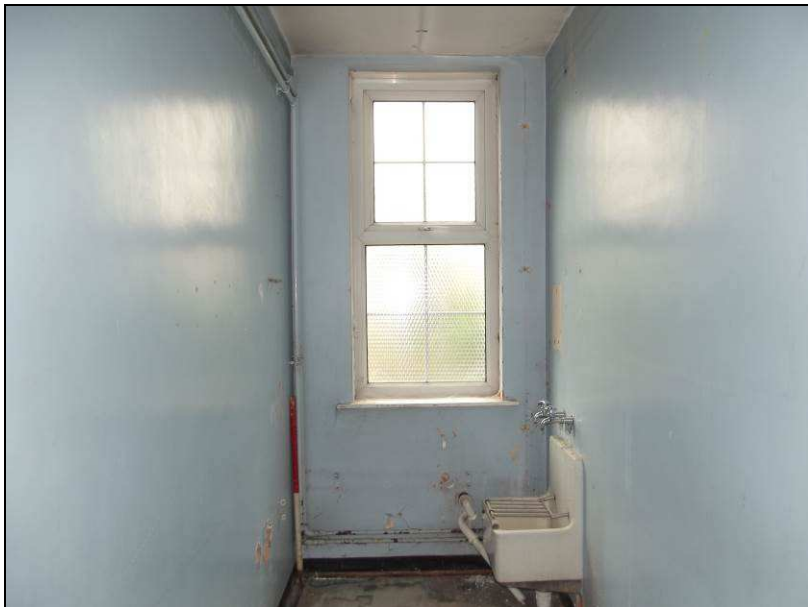
Plate 22 (shot 120): Photo of one of the wash rooms in B6, looking north
