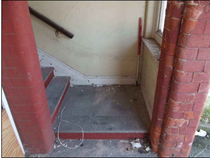
Plate 69 (shot 306): External stairwell on Epworth House. Here bullnose bricks have been used to curve the edges of the doorway, looking southwest
