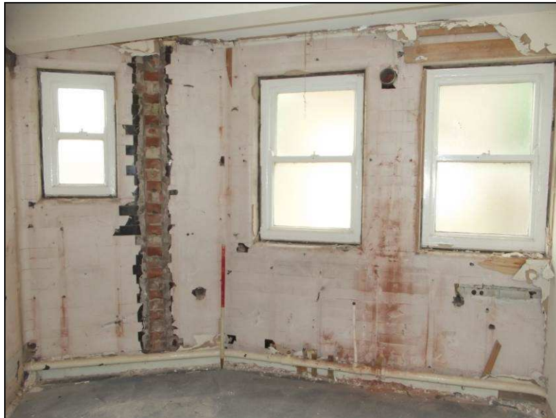
Plate 48 (shot 250): Room in C3 which lacks plastered walls, looking northwest
