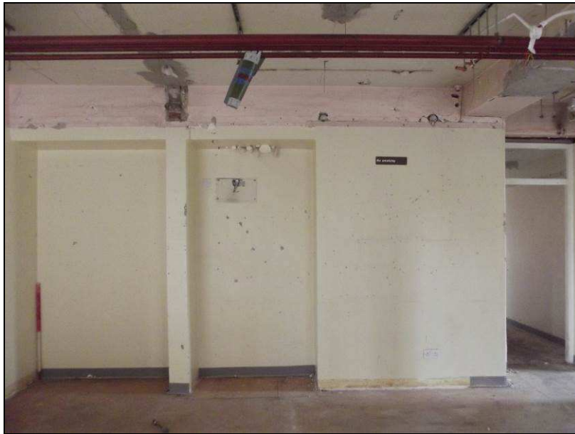
Plate 72 (shot 55): Sealed entrances to part of Epworth House, presumably due to the western extension providing access, looking northeast
