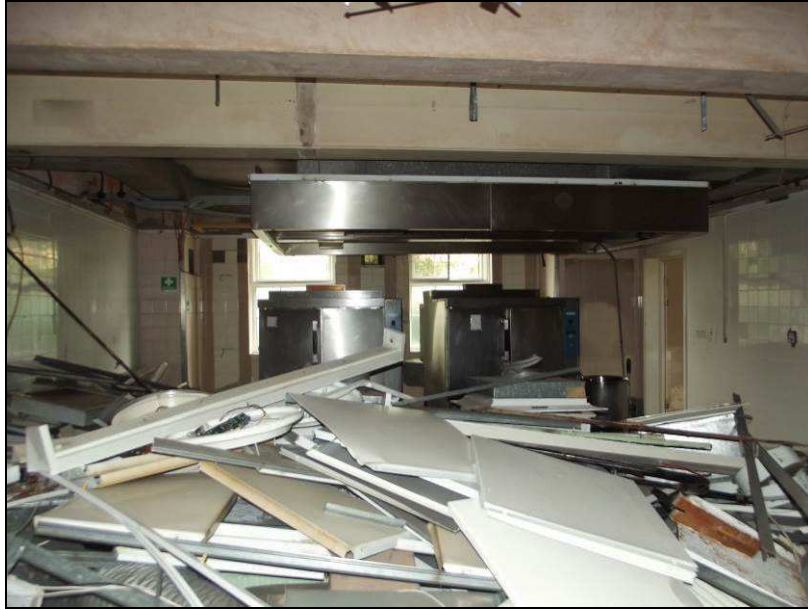
Plate 17 (shot 103): View of catering units in B3, looking north
