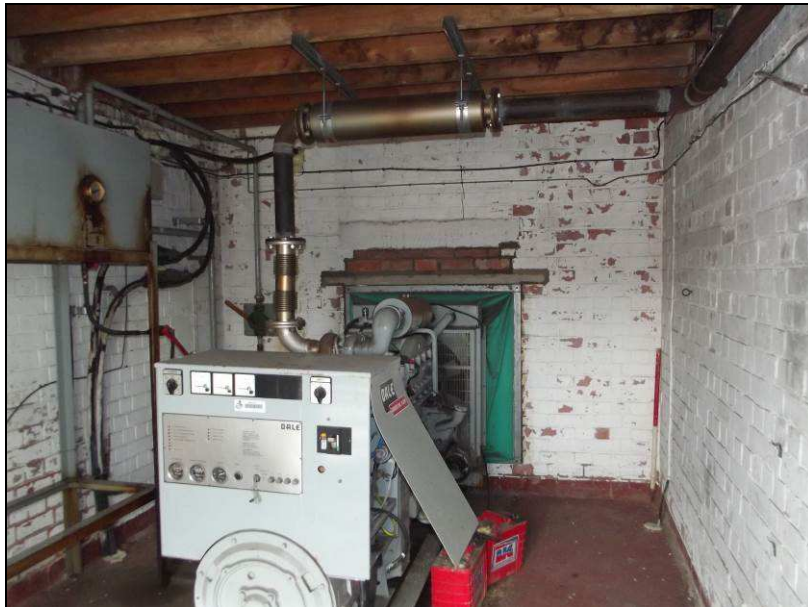
Plate 24 (shot 89): Barton House western extension housing the services for the main building, looking northeast
