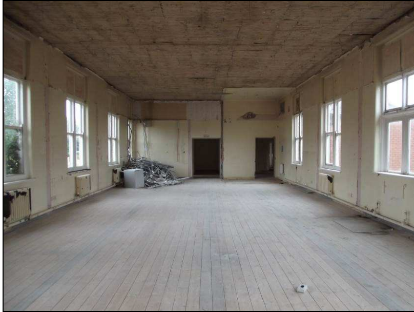
Plate 71 (shot 50): View of the southern half of Epworth House looking northeast. The interior has been stripped of its partitions.
