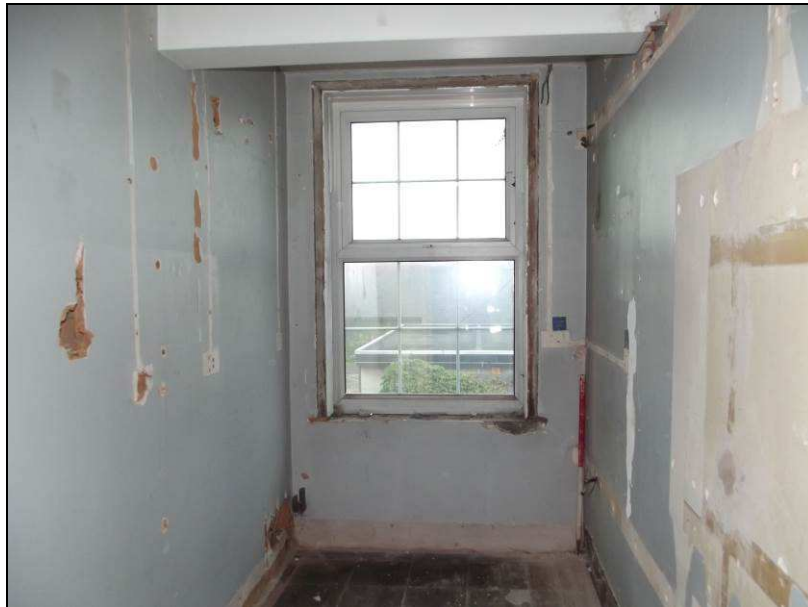
Plate 32 (Shot 170): Small room in B10, possibly used for storage on account of its dimensions, looking south
