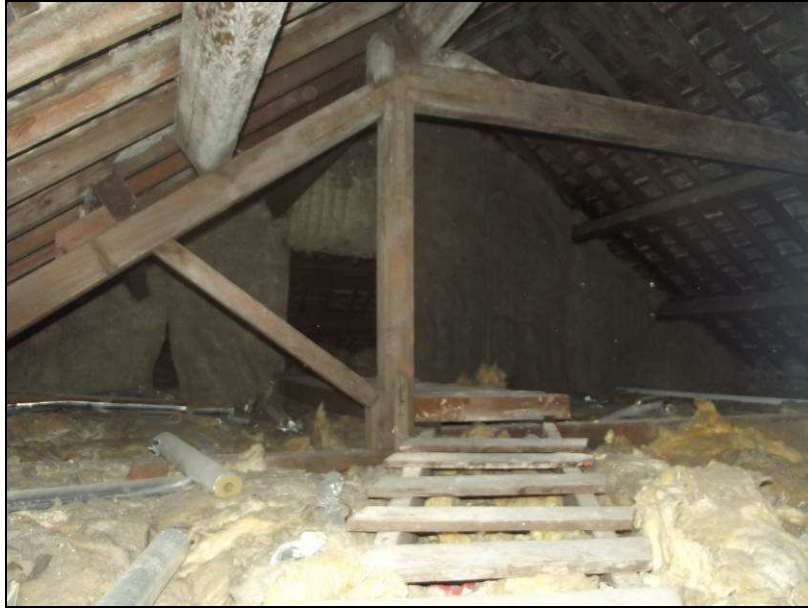
Plate 75 (shot 77): View of the timber roof structure of Epworth House taken from the first floor looking northeast
