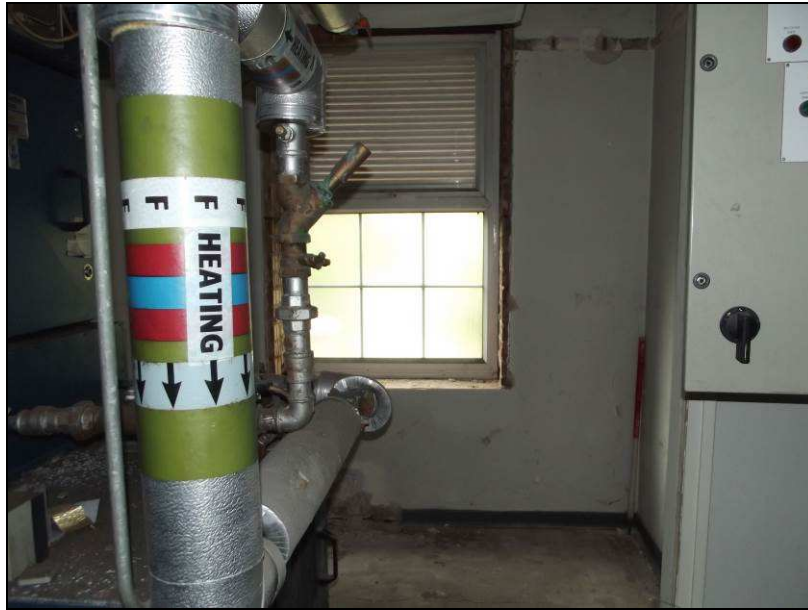
Plate 31 (shot 185): Supply of services to the first floor of Barton House, in B13, looking north
