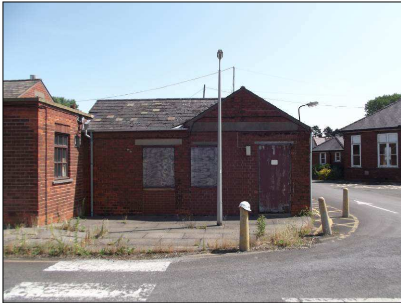
Plate 54 (shot 330): The west facing elevation of the southern extension of Dragonby House, looking east
