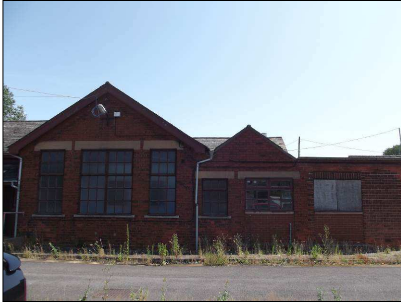
Plate 53 (shot 331): West facing elevation showing an inserted window in the southern extension, looking east
