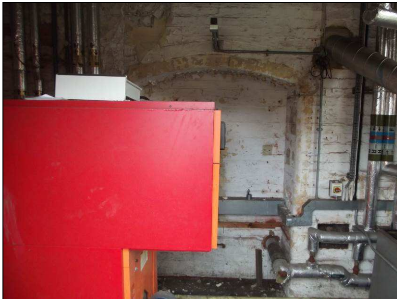
Plate 44 (shot 262): Plant room in Crosby House, looking southeast
