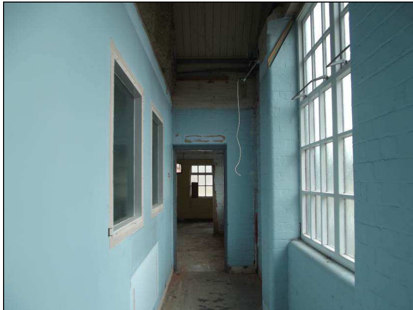
Plate 58 (shot 18): Corridor running down the western extent of the original Dragonby building, looking south
