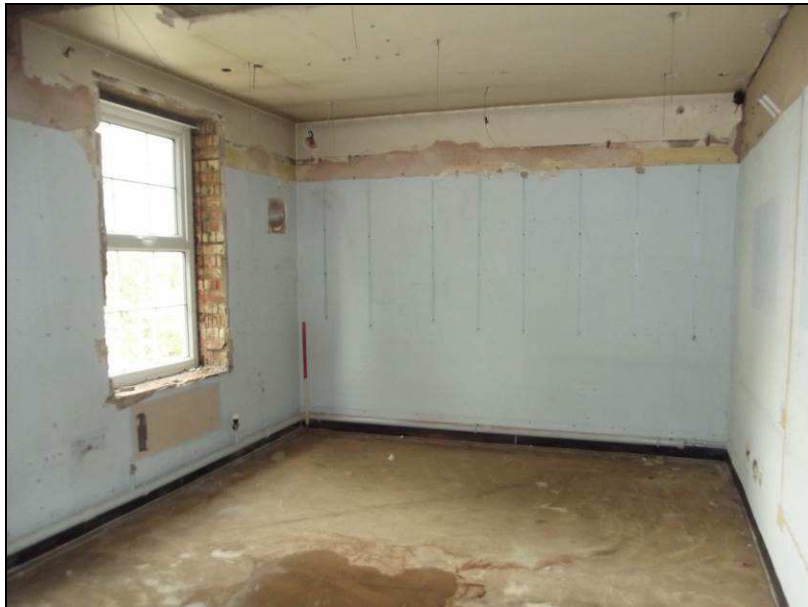
Plate 30 (shot 190): One of the larger rooms on the first floor of Barton House (B12), looking northeast
