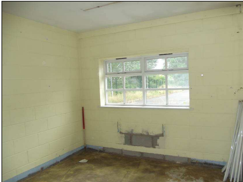
Plate 62 (shot 38): One of three spaces which appear to have been in use as offices or similar in Dragonby House (D4), looking northeast
