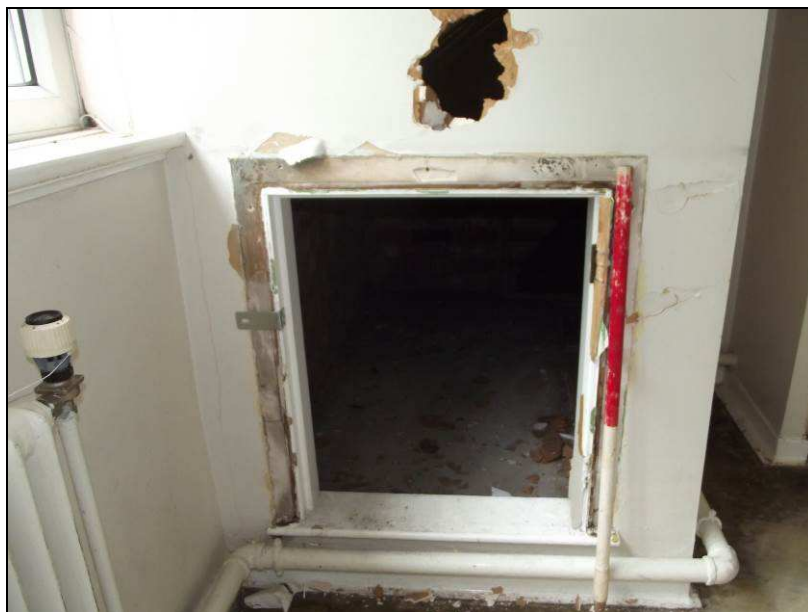
Plate 34 (shot 198): Access point to crawl space behind the outer walls of the second floor of Barton House, looking northeast
