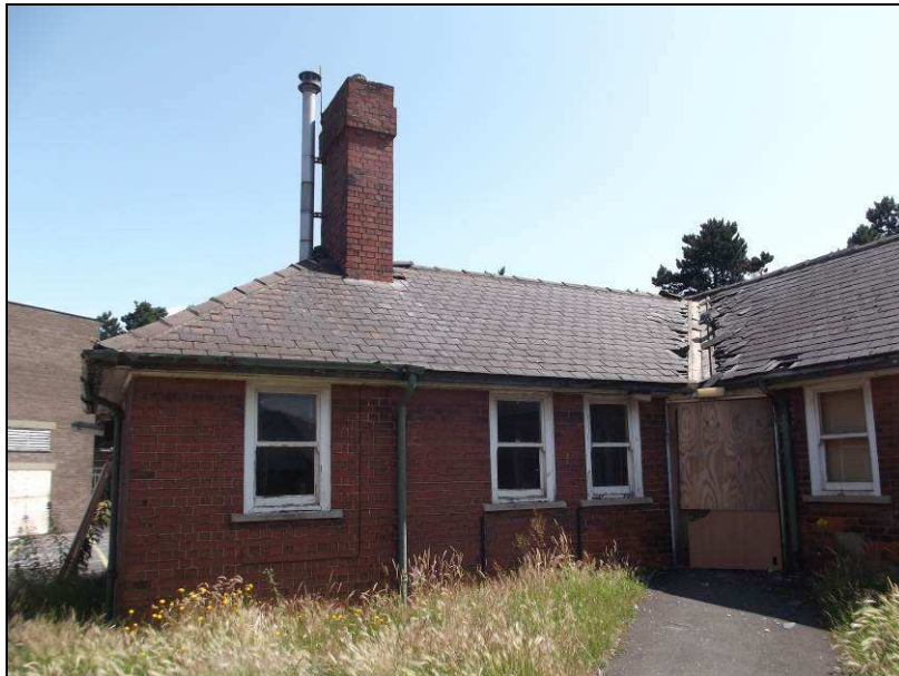
Plate 42 (shot 276): Porch of Crosby House, note the change from stretcher bonding to English bonding either side of the downpipe, looking east
