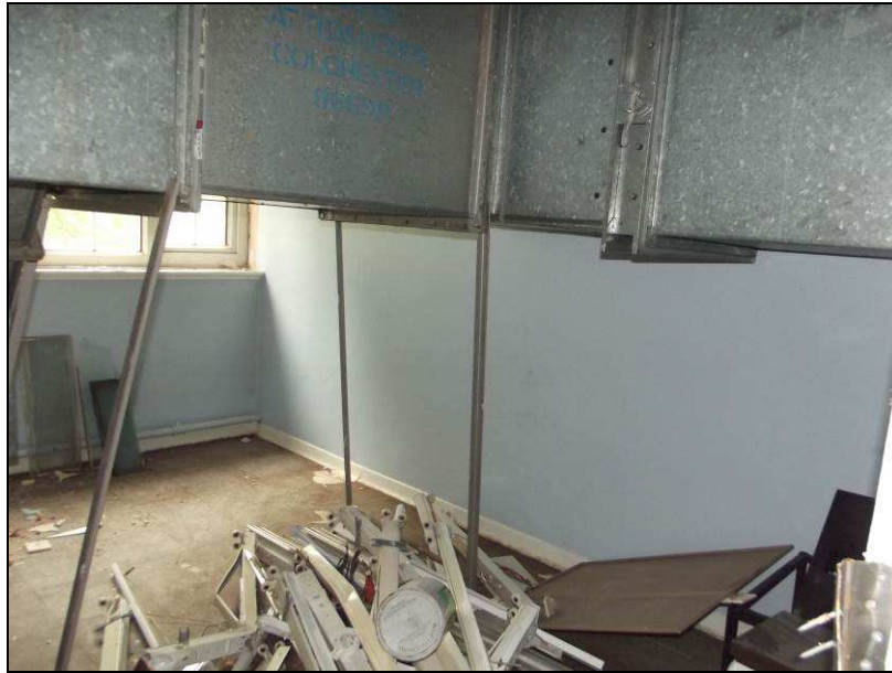
Plate 37 (shot 204): Metal extractors from the lower floors of Barton House found on the second floor, looking northeast
