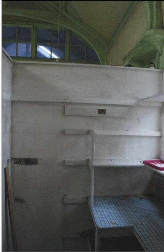
Plate 37 (shot 61): Storage room created by wooden partitions in the kitchen, looking southwest
