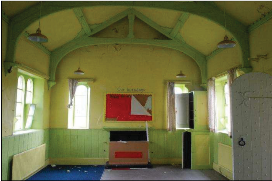
Plate 19 (shot 1): First classroom showing the style of the timber framing, looking southeast, scale 1m
