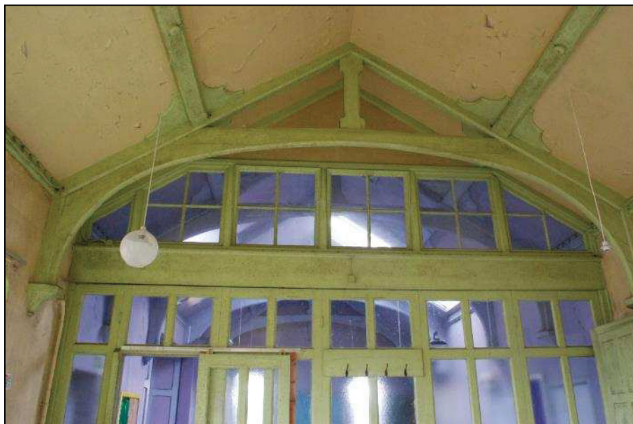
Plate 32 (shot 71): Upper section of partition between school kitchen and classroom, looking southwest
