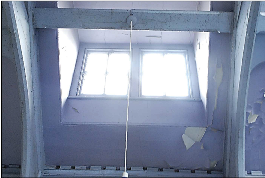
Plate 26 (shot 48): Dormer window inserted into the roof of the southeast elevation, looking southeast
