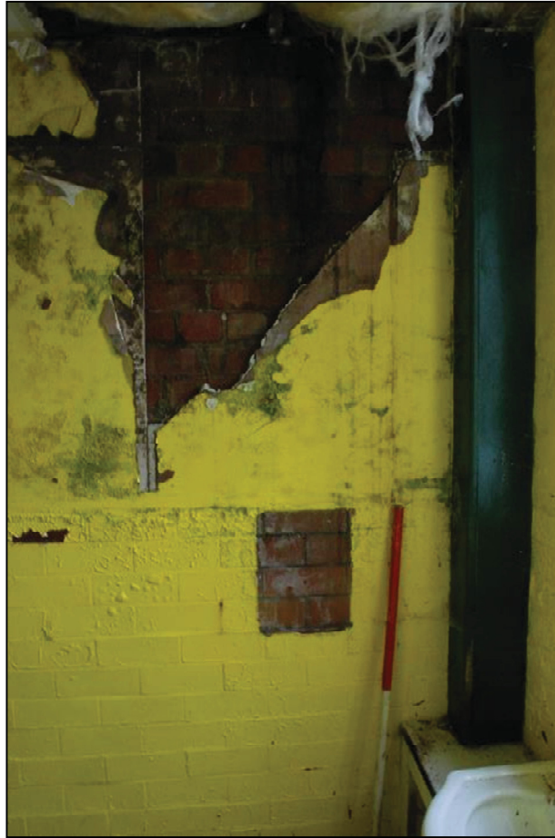
Plate 43 (shot 78): Area of damp in the toilet block, looking northeast, scale 1m
