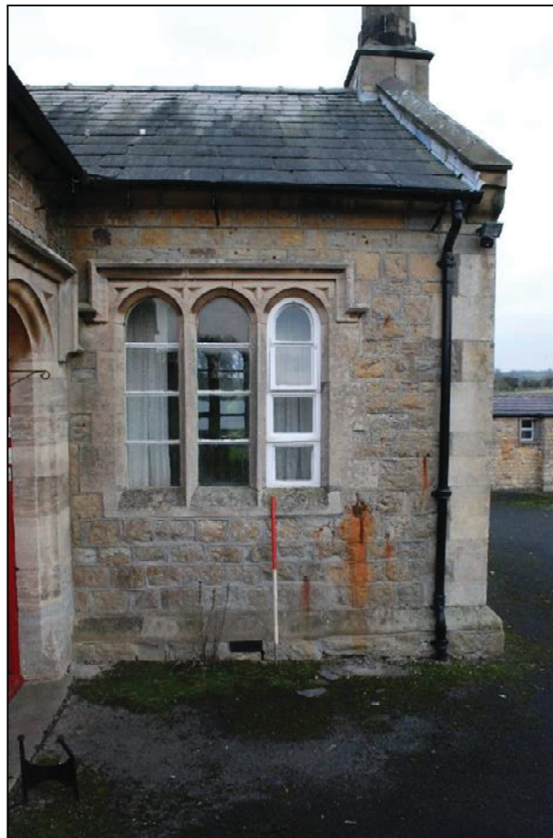
Plate 2 (shot 100): End of the second classroom showing the projecting gable ends and lead flashing, looking northeast, scale 1m
