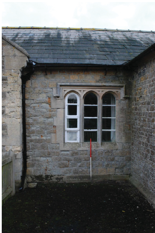
Plate 10 (shot 102): Porch which projects from the second classroom's southwest elevation, looking northeast, scale 1m
