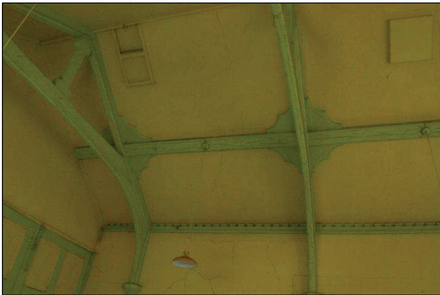
Plate 22 (shot 18): Blocked skylight in the first classroom, looking north
