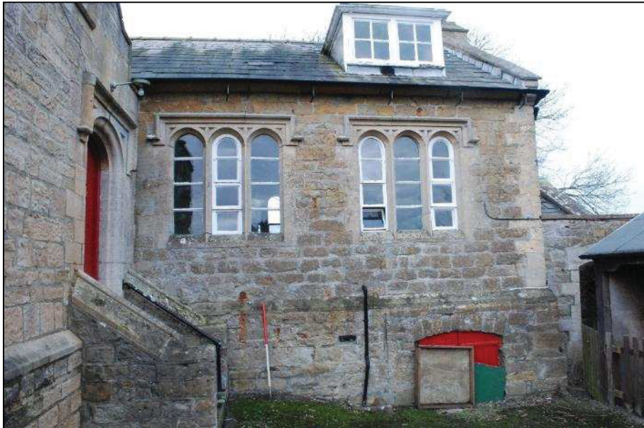
Plate 6 (shot 118): Northeast end of the southeast elevation of the original building, looking northwest, scale 1m
