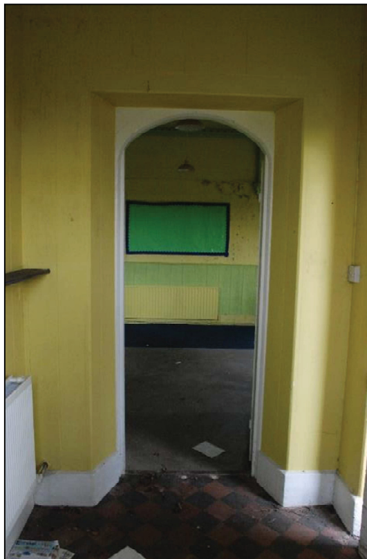
Plate 18 (shot 97): Doorway in northeast elevation leading into the rest of the building, looking northeast
