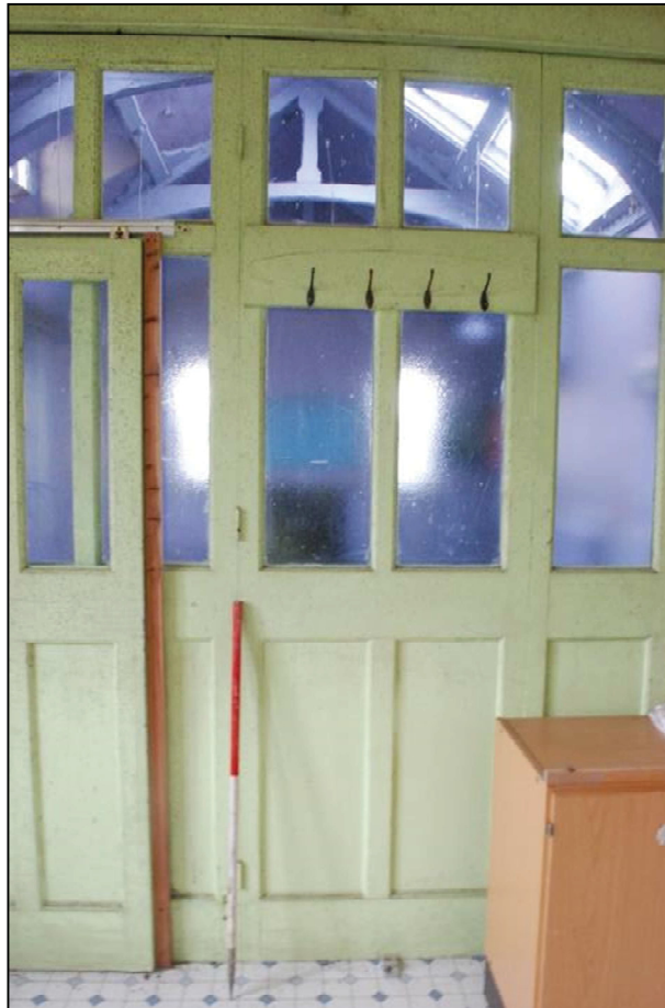
Plate 33 (shot 73): Detail of the folding screen and inserted sliding door, looking southwest, scale 1m
