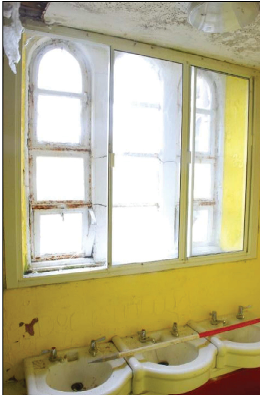
Plate 41 (shot 77): Window and basin on the southeast elevation of the toilet block, looking south, scale 1m
