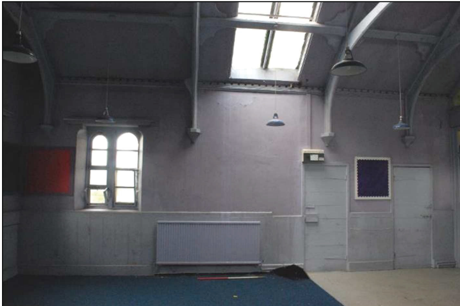
Plate 30 (shot 32): The northwest elevation, two doors to the north are sealed, looking northwest, scale 1m
