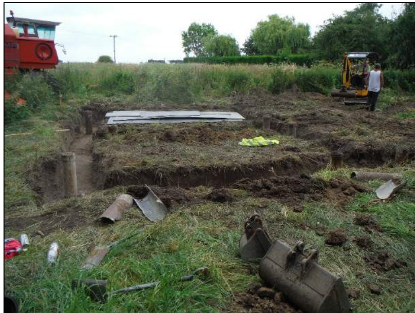
Plate 1: General view of the site looking north, clearly showing concrete piles within the footings
