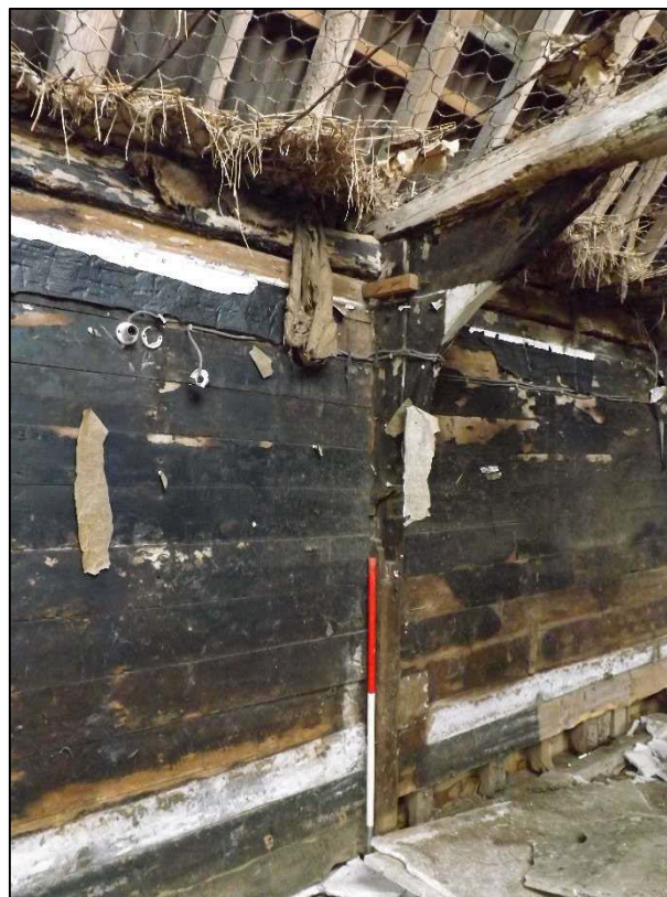
Plate 13 (shot 46): Original tie beam joint to post and wall plate. The joint has been reinforced in a number of places, looking east
