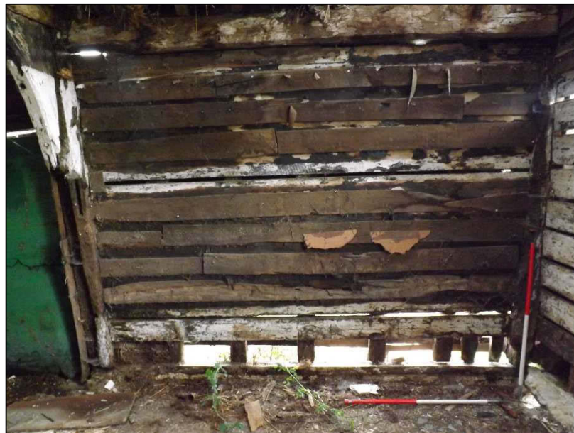
Plate 11 (shot 38): Northern bay of the northeast-facing elevation, studs are visible beneath the weatherboarding, looking southwest
