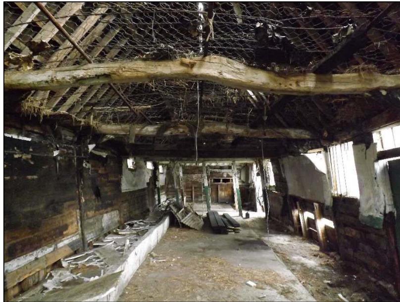
Plate 12 (shot 43): Tie beams at the north end of the building, both are clearly cracked, looking southeast
