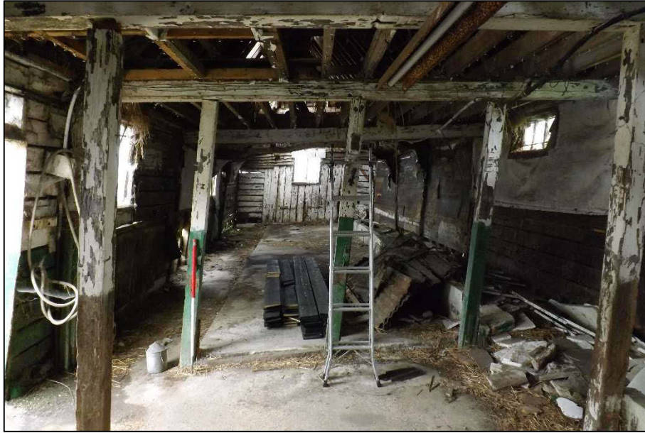
Plate 4 (shot 16): The internal frame is visibly racking. Posts appear to be supporting replacement tie beams, looking northwest
